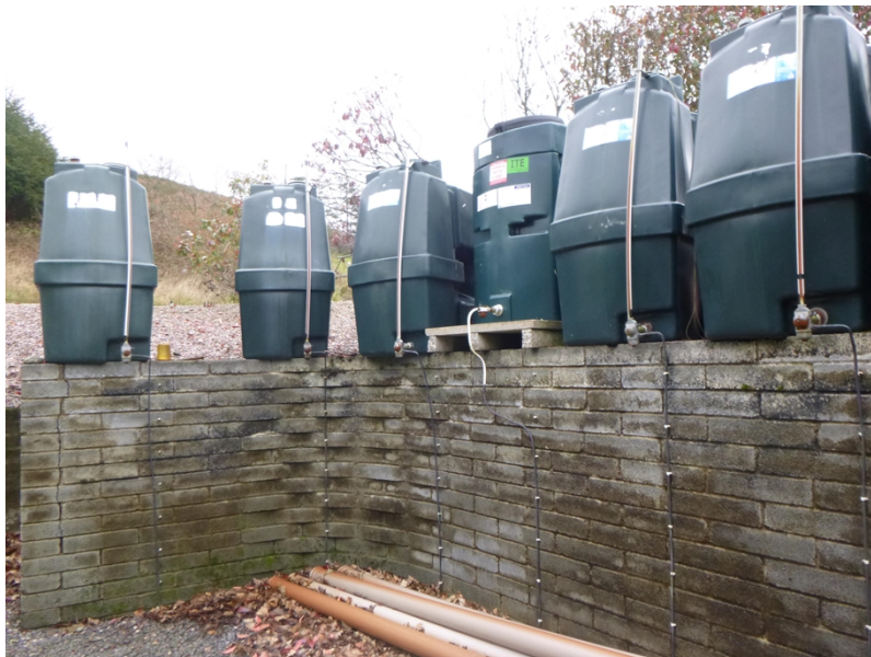
Photograph 2: Oil tanks surrounding Biodisc
