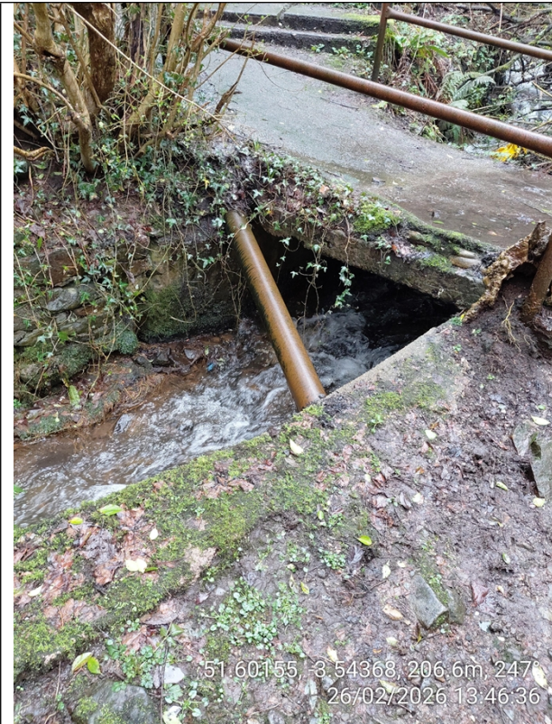
Image 1 - pipework in permitted discharge location
