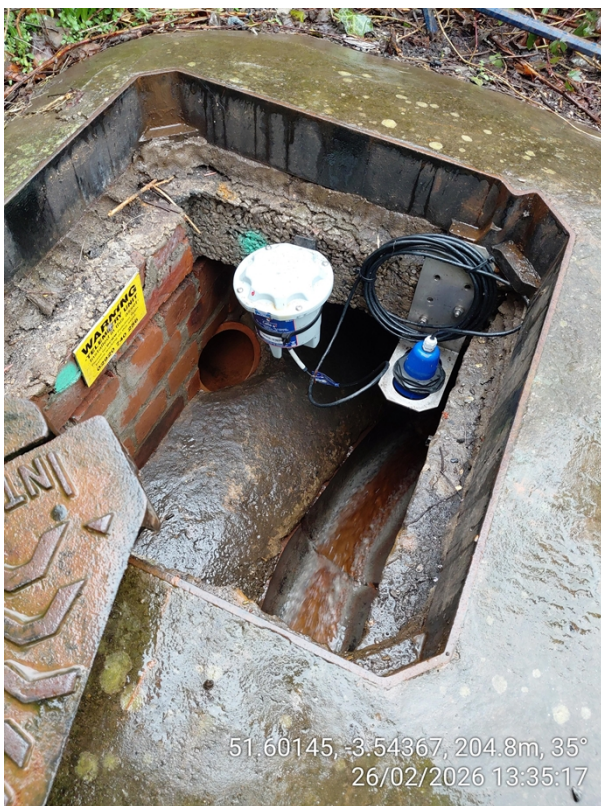
Image 2 - Overflow pipe in chamber
