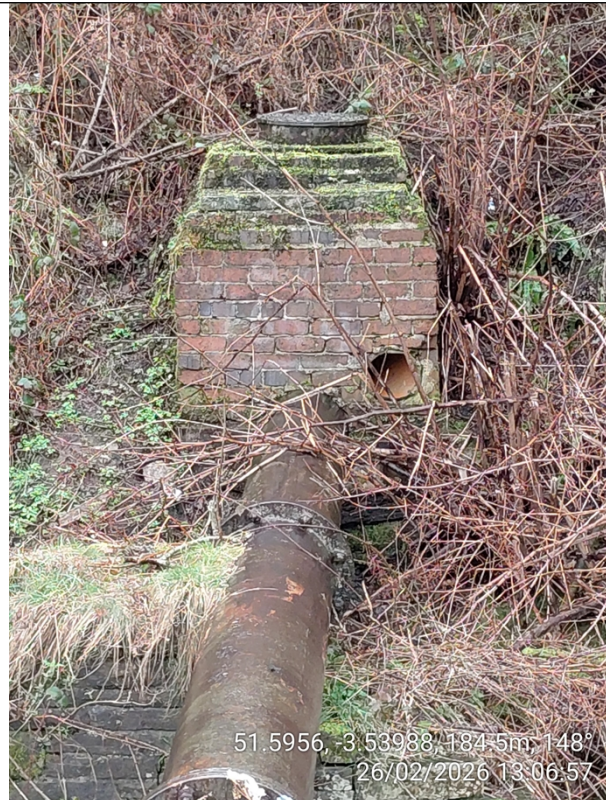
Image 1: Discharge point for CSO
