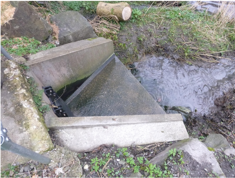
Photograph 1: Outfall at Tregaron SPS
