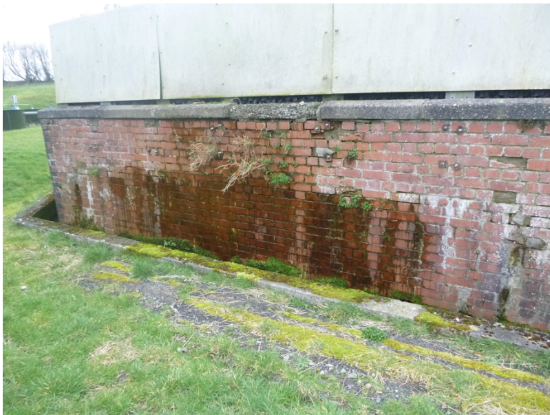
Photograph 2: leaking filter bed
