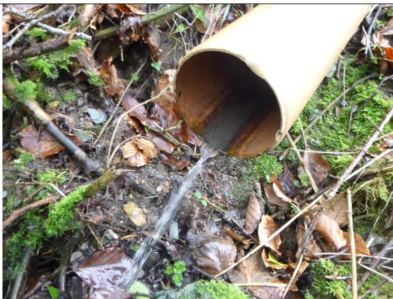
Photograph 3: Final effluent discharge
