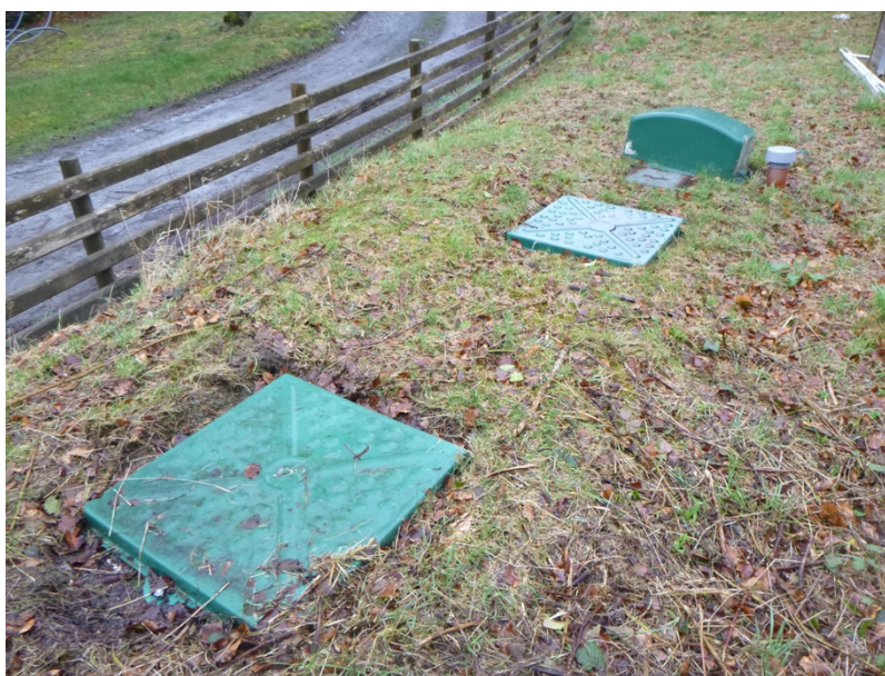
Photograph 1: Package Treatment Plant (PTP)
