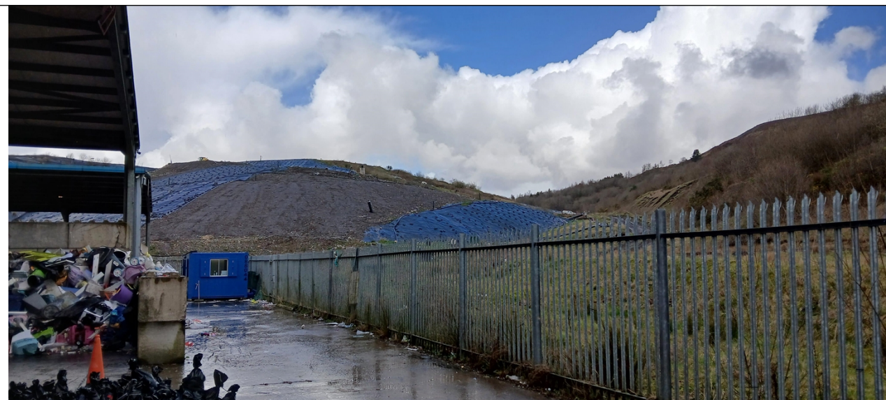
Photo 6 - Taken from the waste transfer station of the Bryn Pica Landfill active tipping face with, at the time of visit, approx. 30% of temporary capping installed
