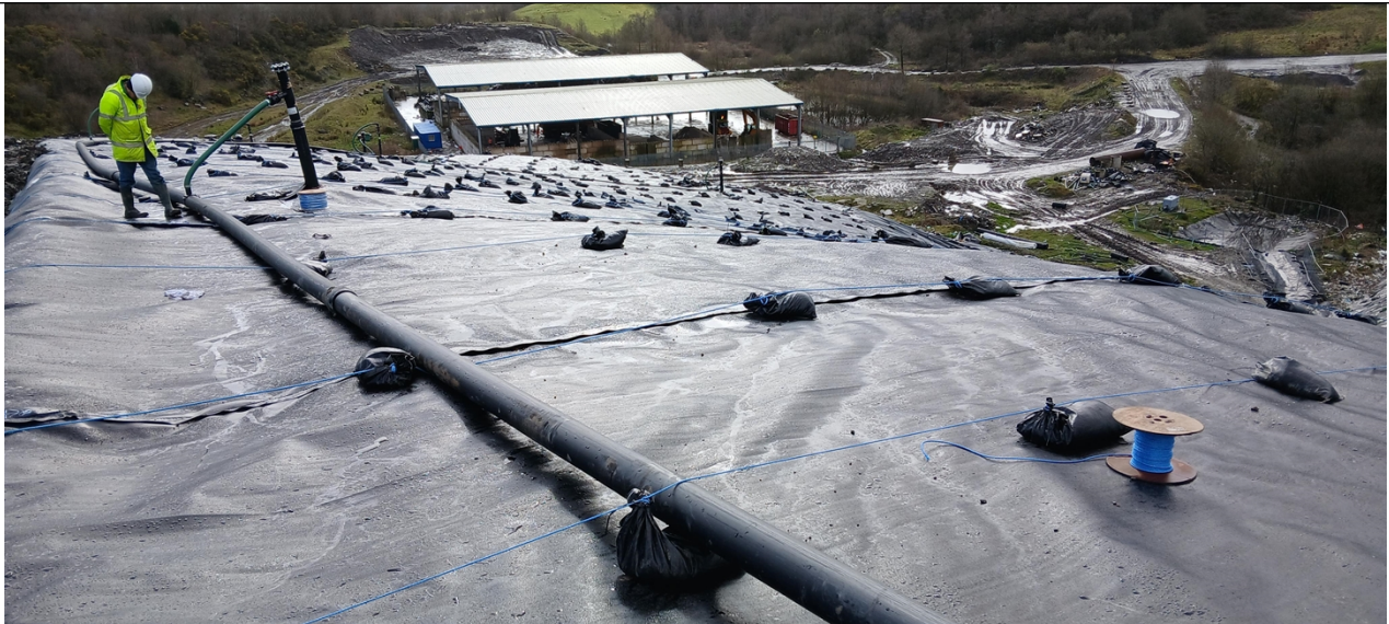
Photo 3 - Installed temporary capping on active tipping face at Bryn Pica (photo taken on 13/03/26)
