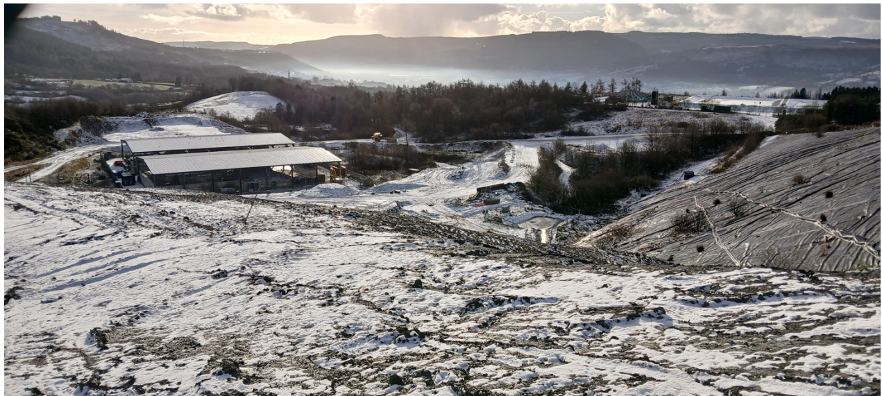
Photo 2 - Active tipping face at Bryn Pica with no temporary capping installed (photo taken on 06/01/26)
