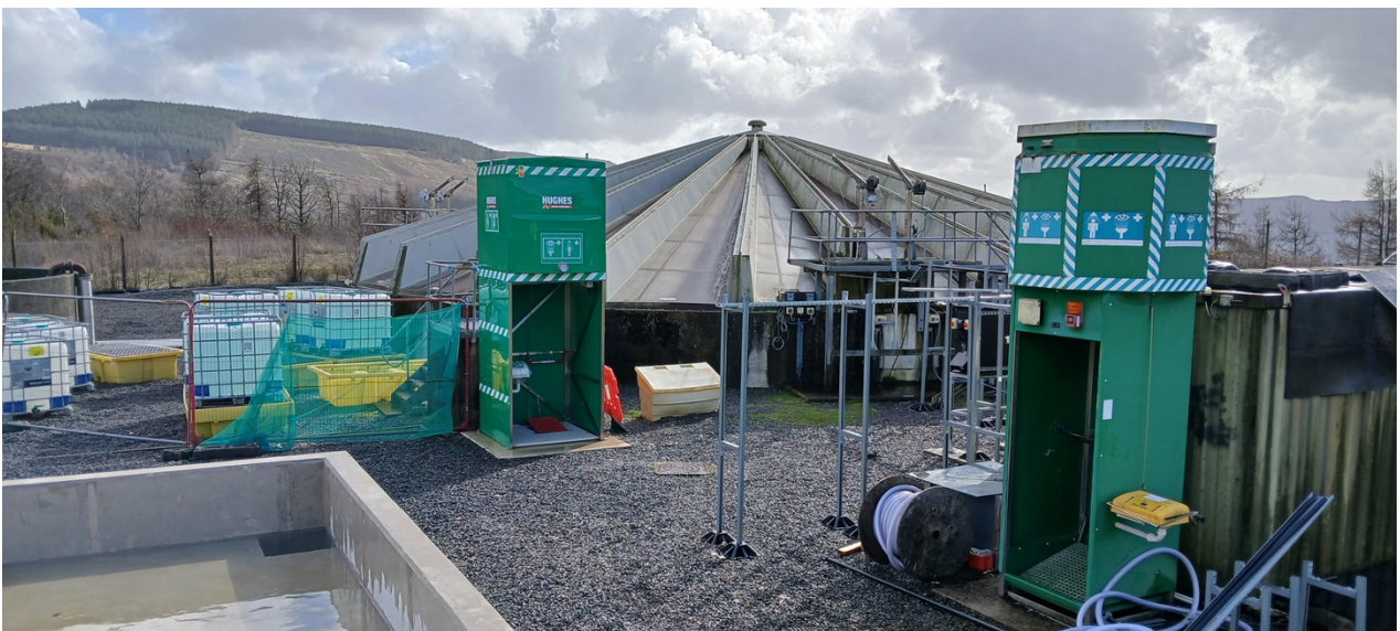
Photo 5 - Leachate treatment tank at Bryn Pica Landfill
