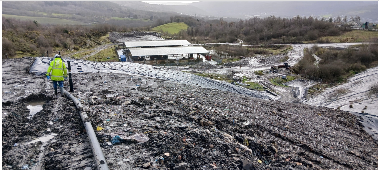
Photo 1 - Installed temporary capping on active tipping face at Bryn Pica (photo taken on 13/03/26)
