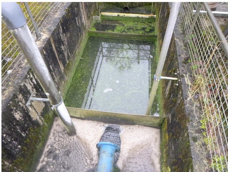
Photograph 4: Final settlement tank
