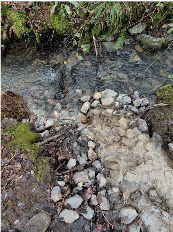
Photograph 3 - The point of Ingress at the end of the channel (Point of Discharge 2) into
