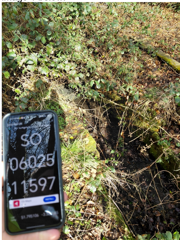
Image 1: One of the discharge locations from the lagoon - other discharge point not seen during the visit.
