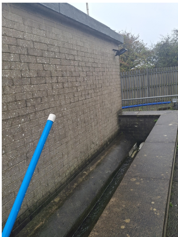
Figure 3: Final Effluent sampling point (unmarked)
