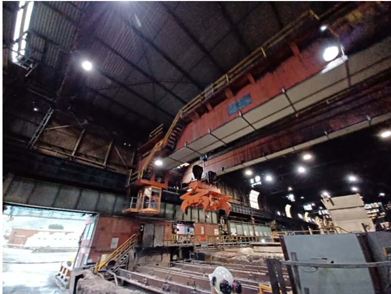
Image 4: View of faulty Middle Outer Crane (AA146) associated with the Hot Rolling Mills
