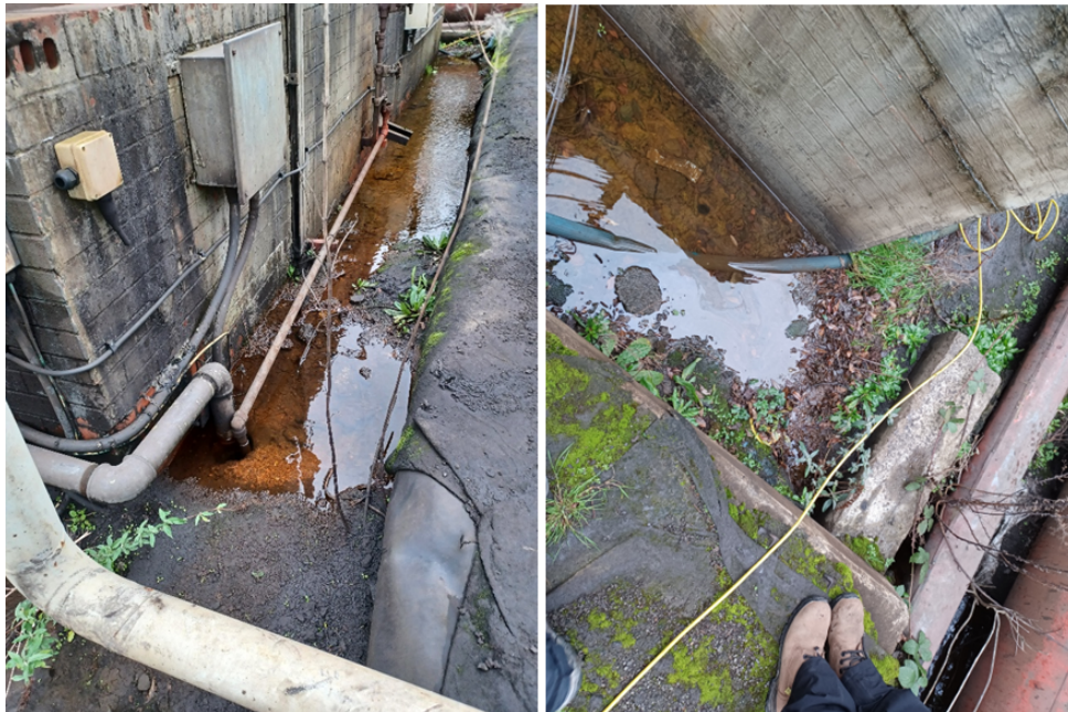
Image 2 & 3: Outlet pipe associated with Latex Tank appeared to be flooded, allowing for a release of water to ground behind the bund.
