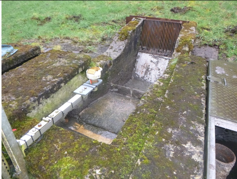
Photograph 1: Inlet storm overflow
