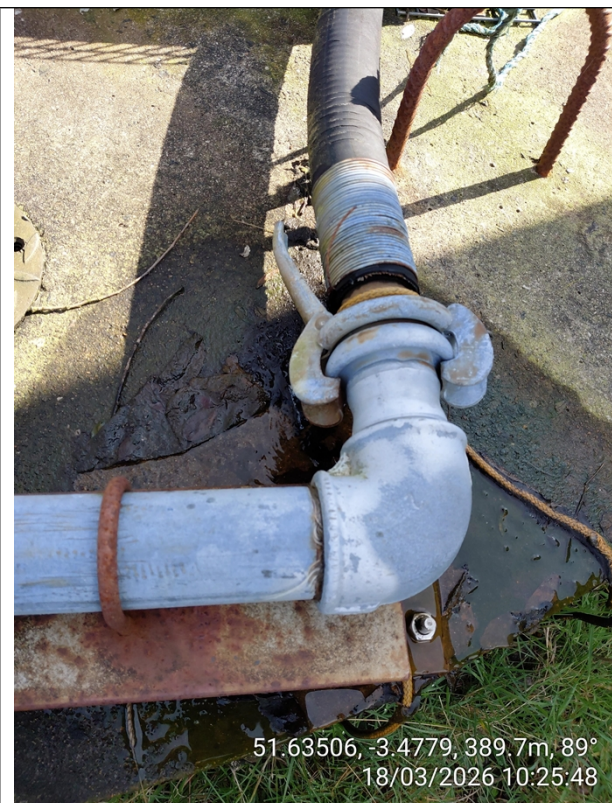
Image 3: leak from leachate pipework
