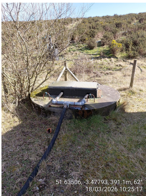
Image 1: leachate pump chamber
