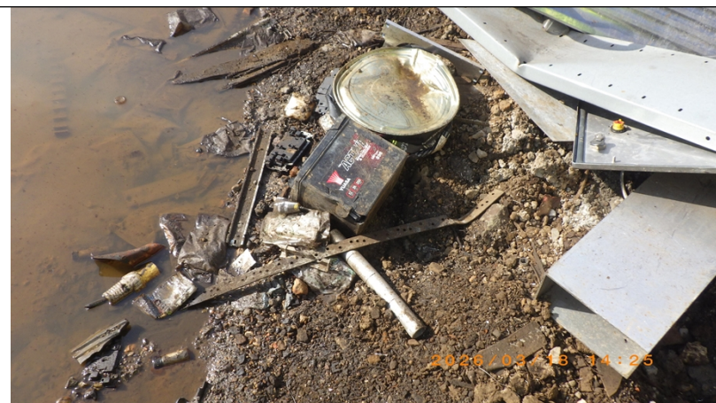
Photograph of battery not stored in required lidded container
