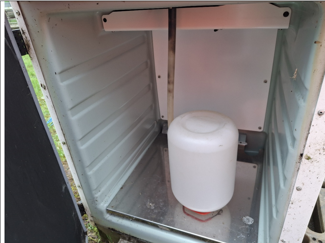
Image 4: Final effluent Aquamatic sampling machine hose with slime build up.
