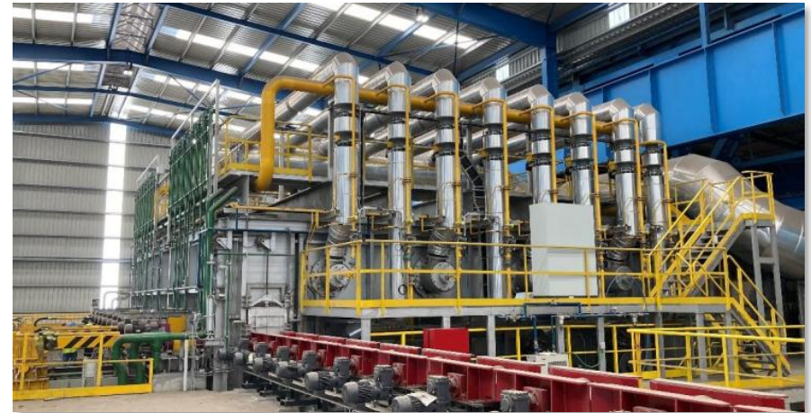
Photograph 1: Replacement furnace (Source: https://www.fivesgroup.com/ )
