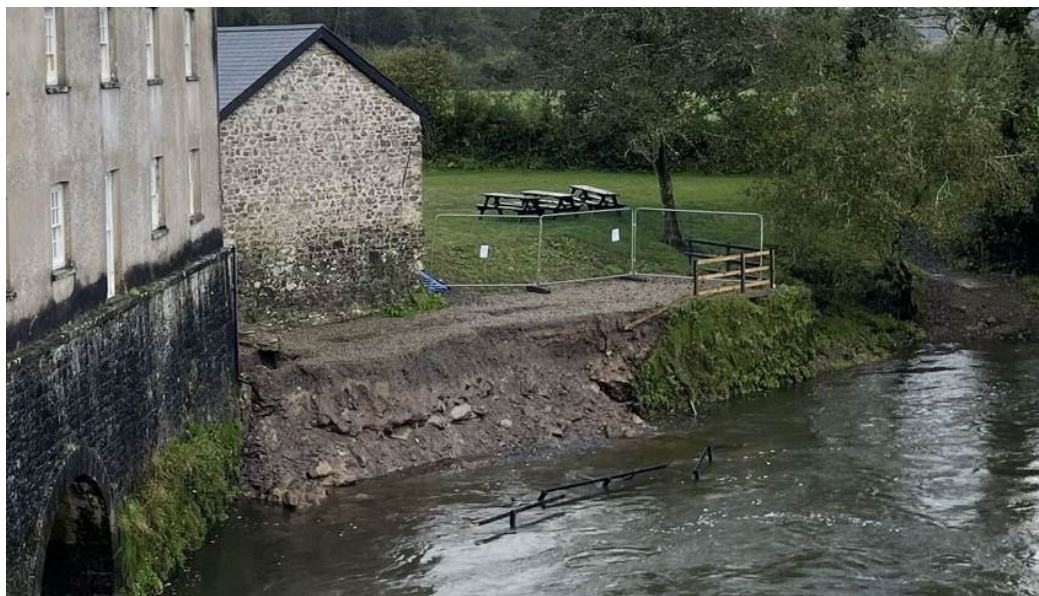
Figure 1: The riverbank wall photographed post-collapse in 2023
