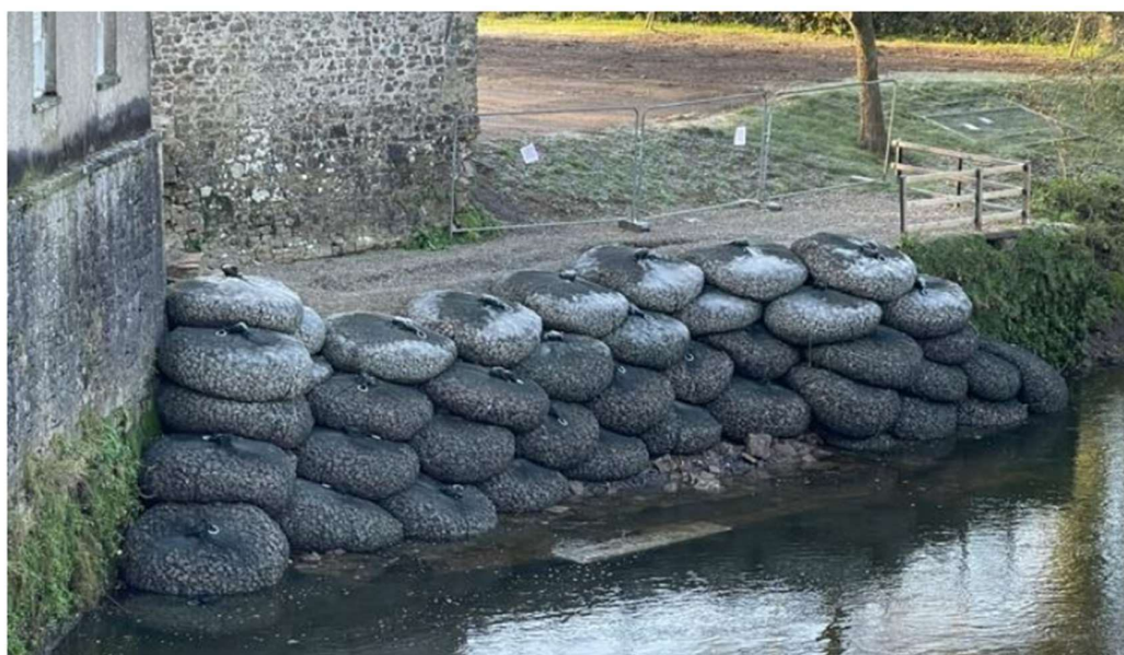
Figure 2: Emergency stabilisation works on the riverbank wall at Black Pool Mill - 48 x Salix Aqua Rock Bags (placed in November 2023)
