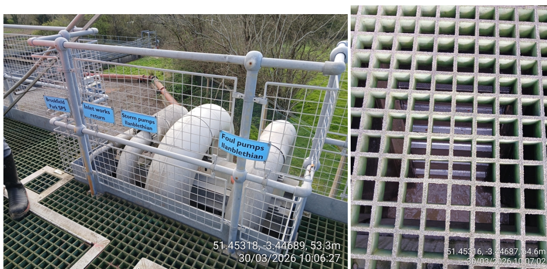
Left: Inlet pumps. Right: Inlet screens.
