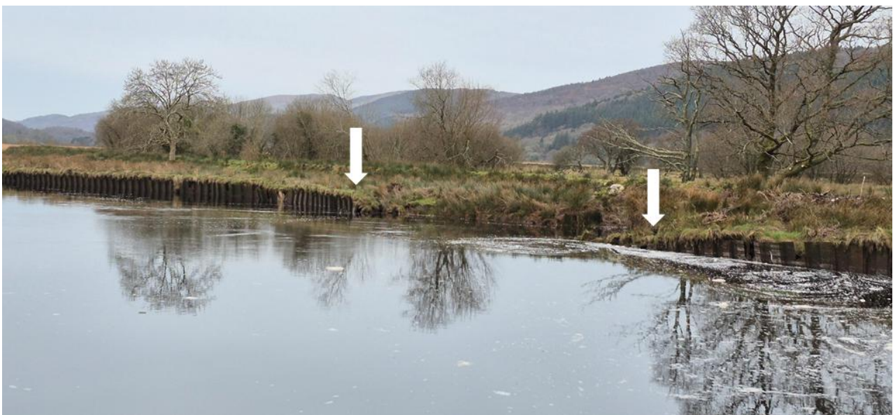
Figure 3-3 Shows the section of failed sheet piling (between white arrows) on the Afon Mawddach (right bank looking downstream, SH 71235 19076)
