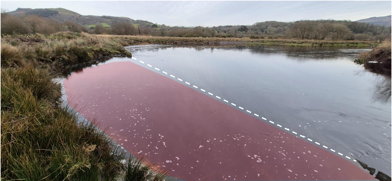
Figure 3-4 Shows the section of failed sheet piling and the extent of subsequent lateral channel movement and scour. White line represents where the existing bank line and sheet piling was. With the red area representing the extent of scour (right bank looking upstream, SH 71174 19069).
