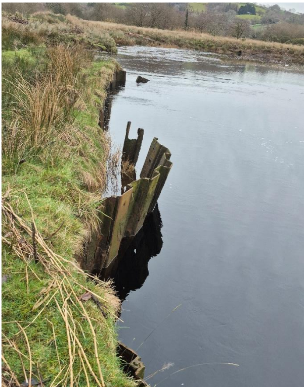
Figure 3-5 The downstream section of sheet piling beginning to fail (right bank looking upstream).
