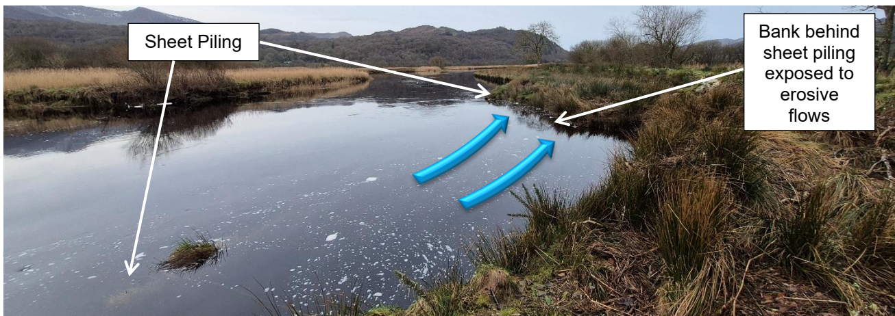
Figure 4-1 Shows how erosive flows can be directed to the bank behind the downstream sheet piling (flow is represented in blue arrows) (photo take from right bank looking downstream)
