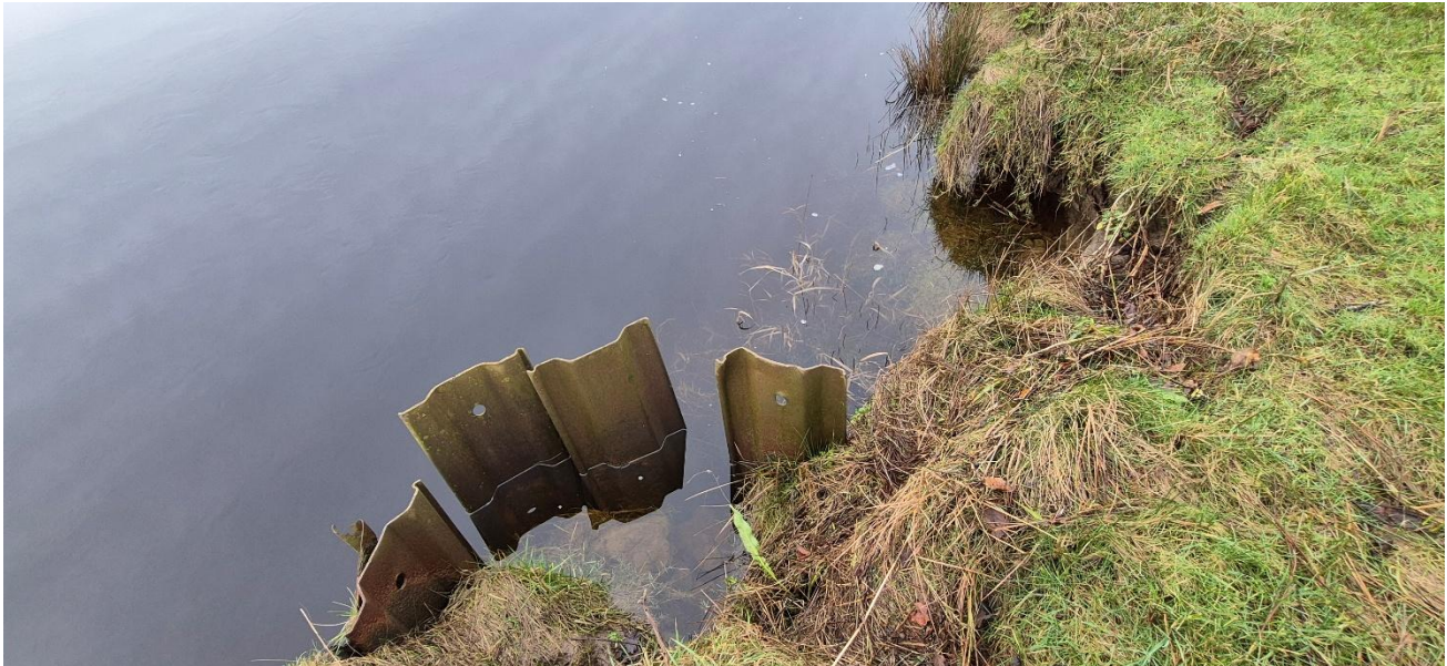
Figure 3-11 Evidence of basal scour and slumping causing deterioration and failure of the sheet piling at the downstream end of the site (right bank looking downstream)
