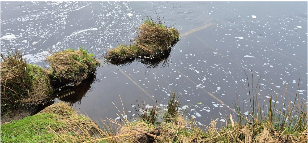
Figure 3-4 Foundation tie rods of the failed sheet piles still in place, just visible below the high tide (right bank looking downstream)
