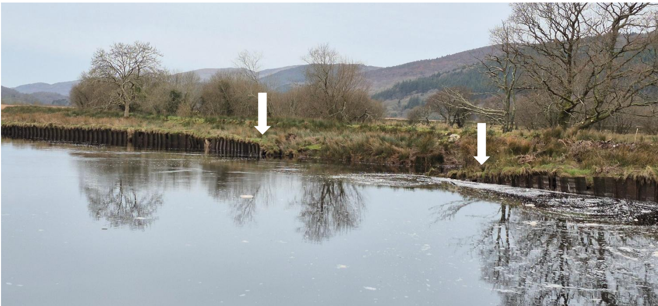
Figure 3-1 Section failed sheet piling in the middle of the image between the white arrows (Left bank looking downstream)
