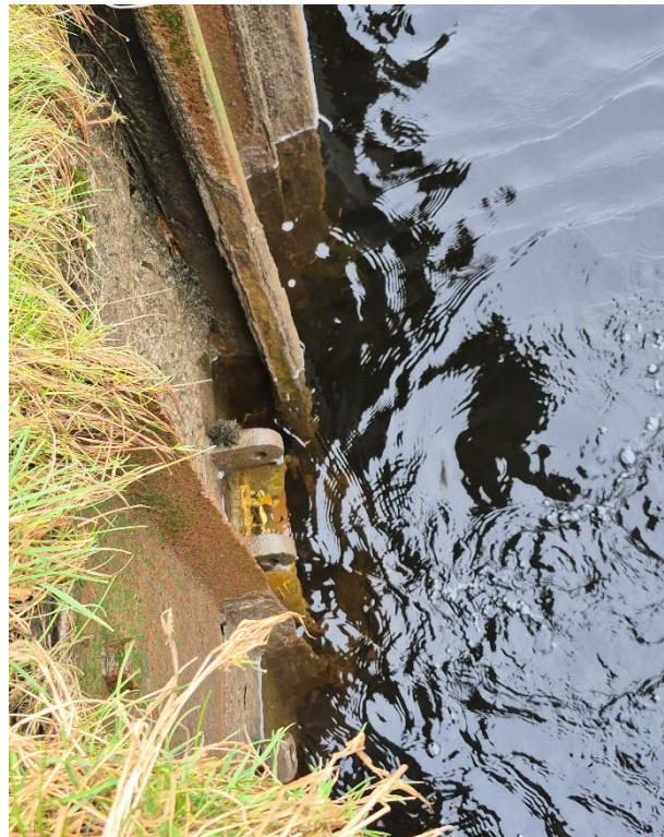
Figure 3-6 Outfall in the sheet piling missing a flap valve (right bank looking upstream).
