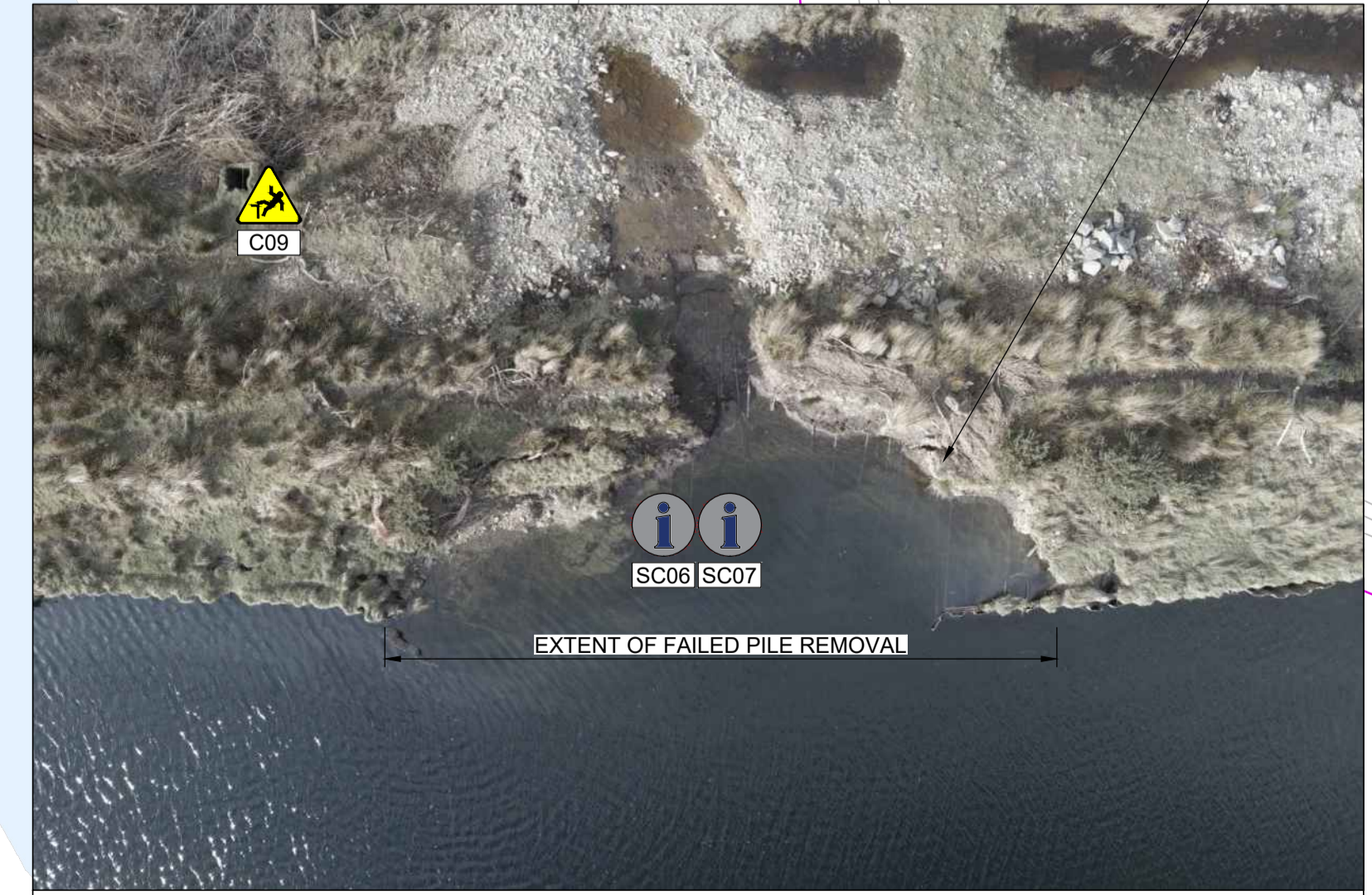
FIGURE 1 BANK SLIP AND FAILED PILES
