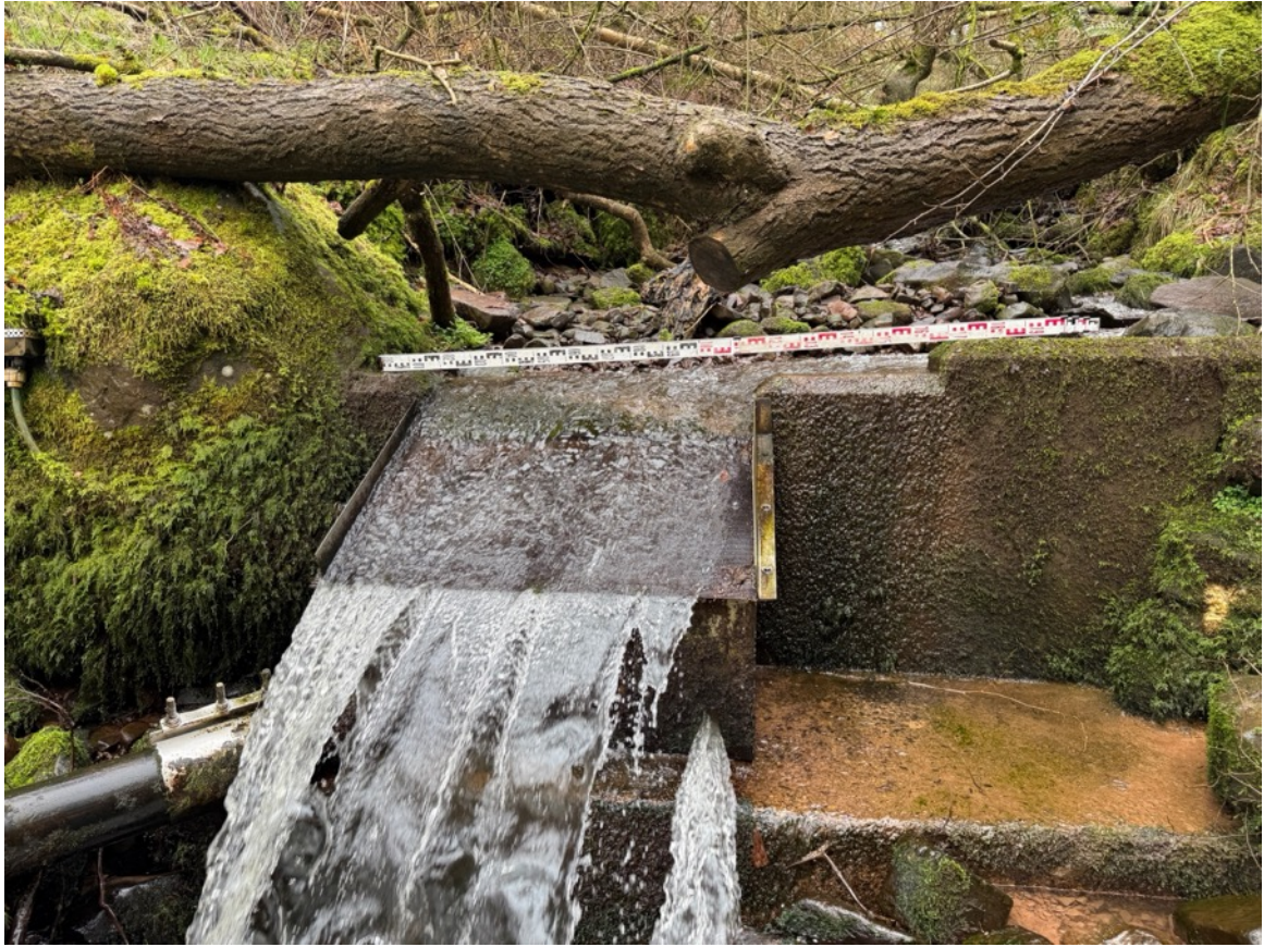
Photo 2f – Looking west up the main stream and at the face on the existing intake structure. Previous hands off flow achieved through calibrated hole in bottom right of the intake box.
