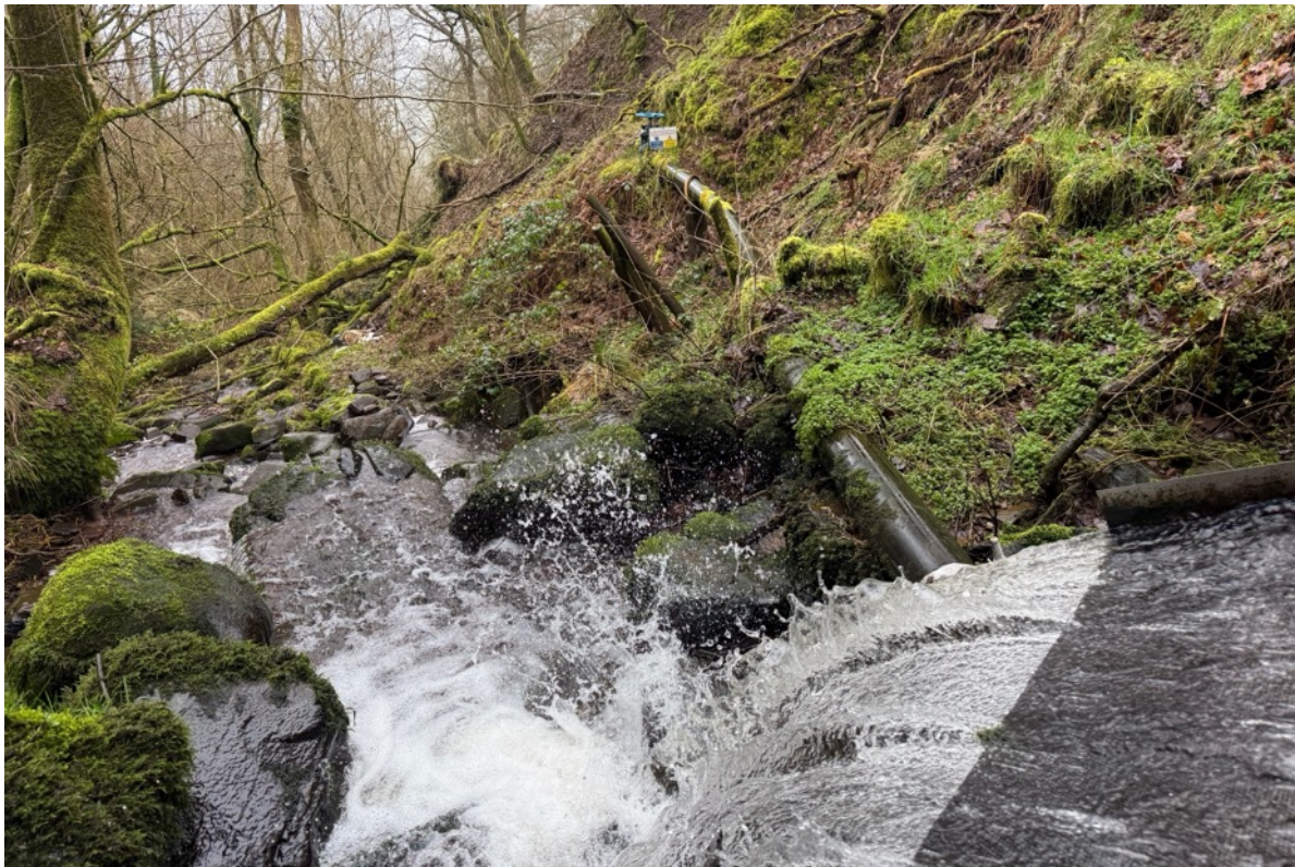
Photo 2e – Looking east down the main stream, from on top of the intake. Intake box in bottom right and penstock leaving box cutting above ground across the slope on the right.
