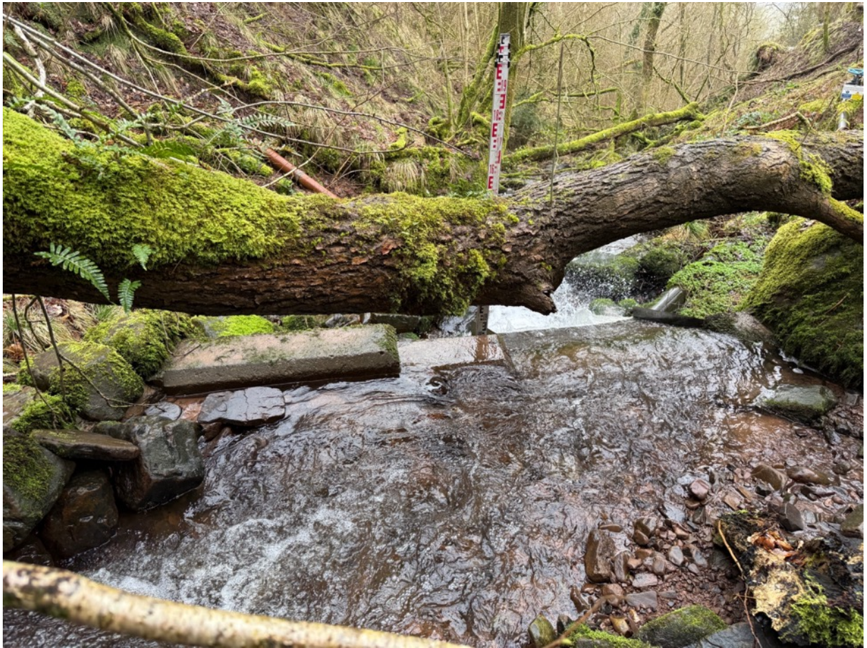
Photo 2d – Looking east over the intake wall and down the main stream.
