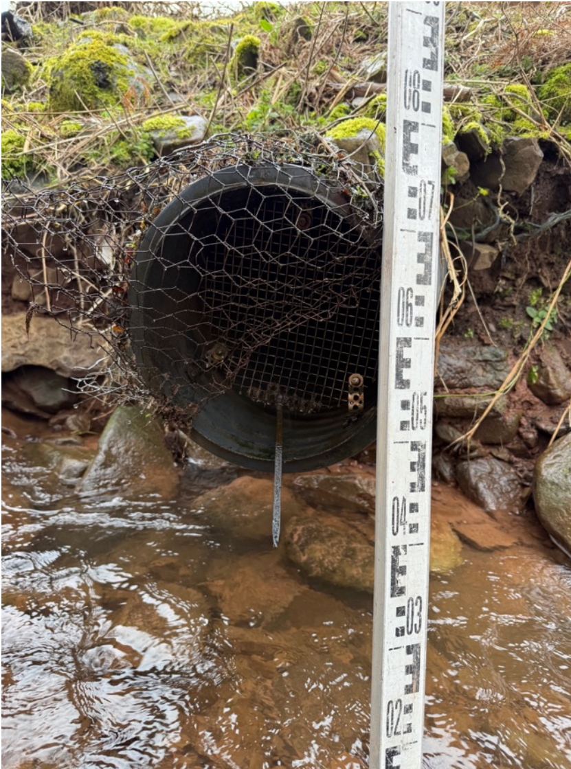
Photo 13d – Existing/proposed outfall pipe showing 10mm mesh within pipe.
