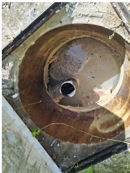
Figure 2: Final effluent chamber
