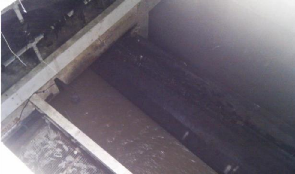
Figure 5: Internal View of Screen Chamber
