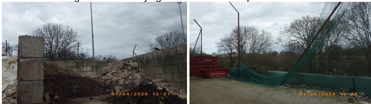
Areas of damaged netting ACTION: Repair damaged netting by Friday 22nd May 2026
