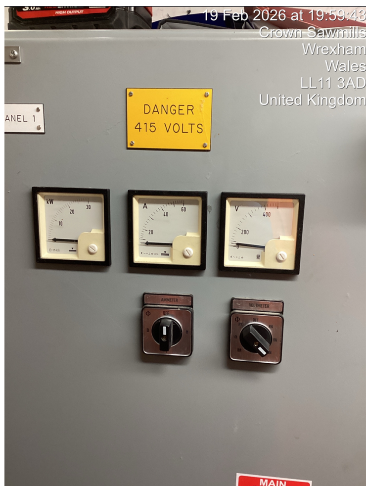
Photo of mains incomer with no amps.
