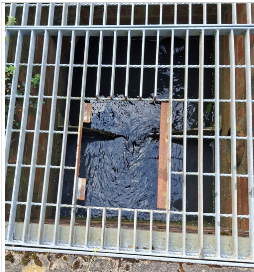
Photo 2: V-notch sample point showing signs of flooding and VOG
