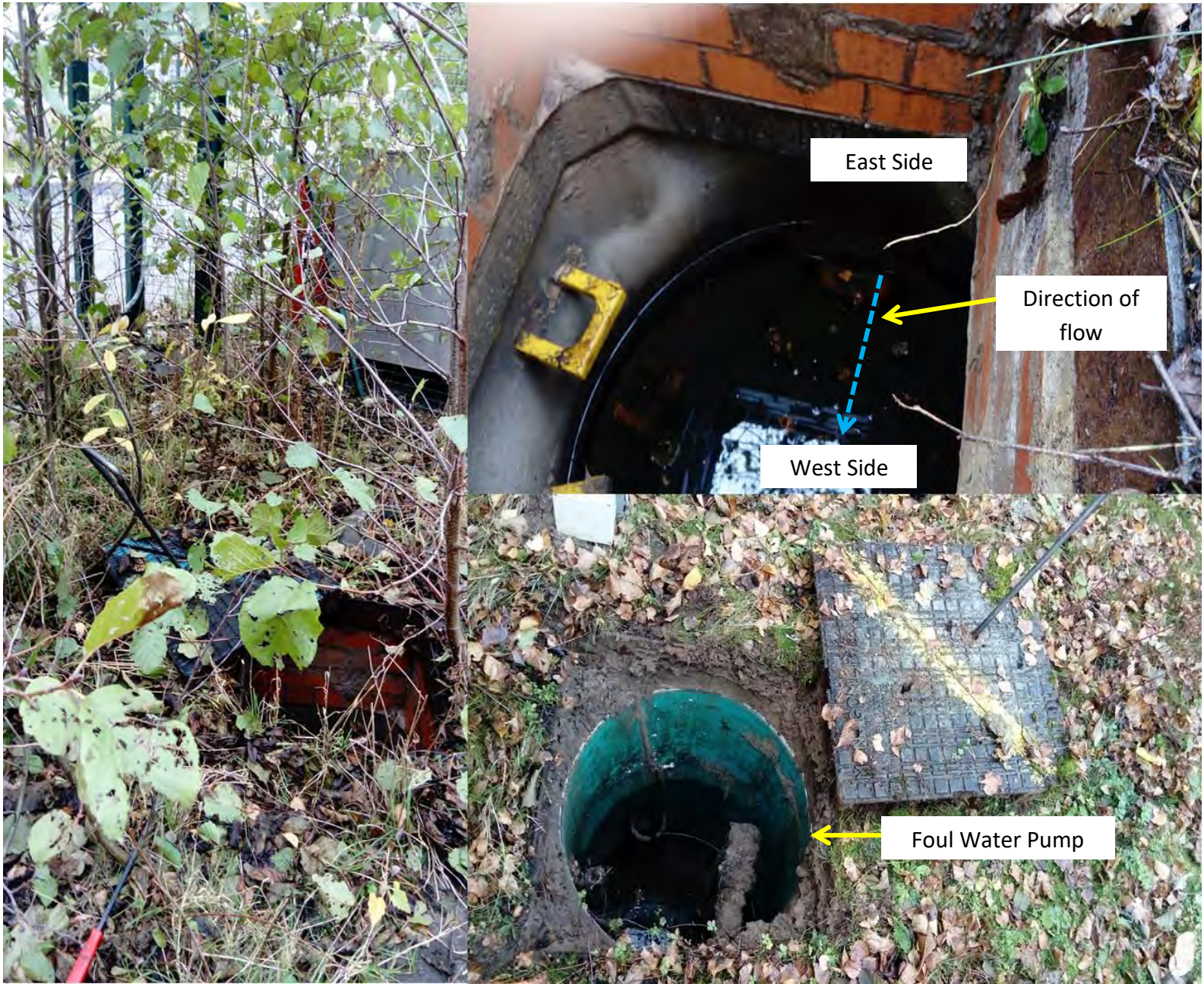
Photograph 7 – Surface water drainage and Foul water pump adjacent to site access gate. Surface water draining in a westwards direction towards the culvert at Weighbridge Rd.
