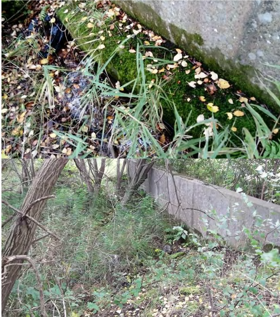
Photograph 9 –Blocked culvert under Weighbridge Rd, near site main access gate. Silted-up and overgrown downstream watercourse receptor.
