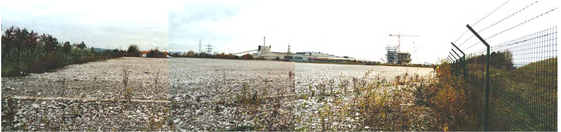
Photograph 22 – Looking North-westwards on to on demolish hard-core area of Shotton Power Station at the south-eastern corner of undeveloped area of the site. Construction of new EfW facility in background.
