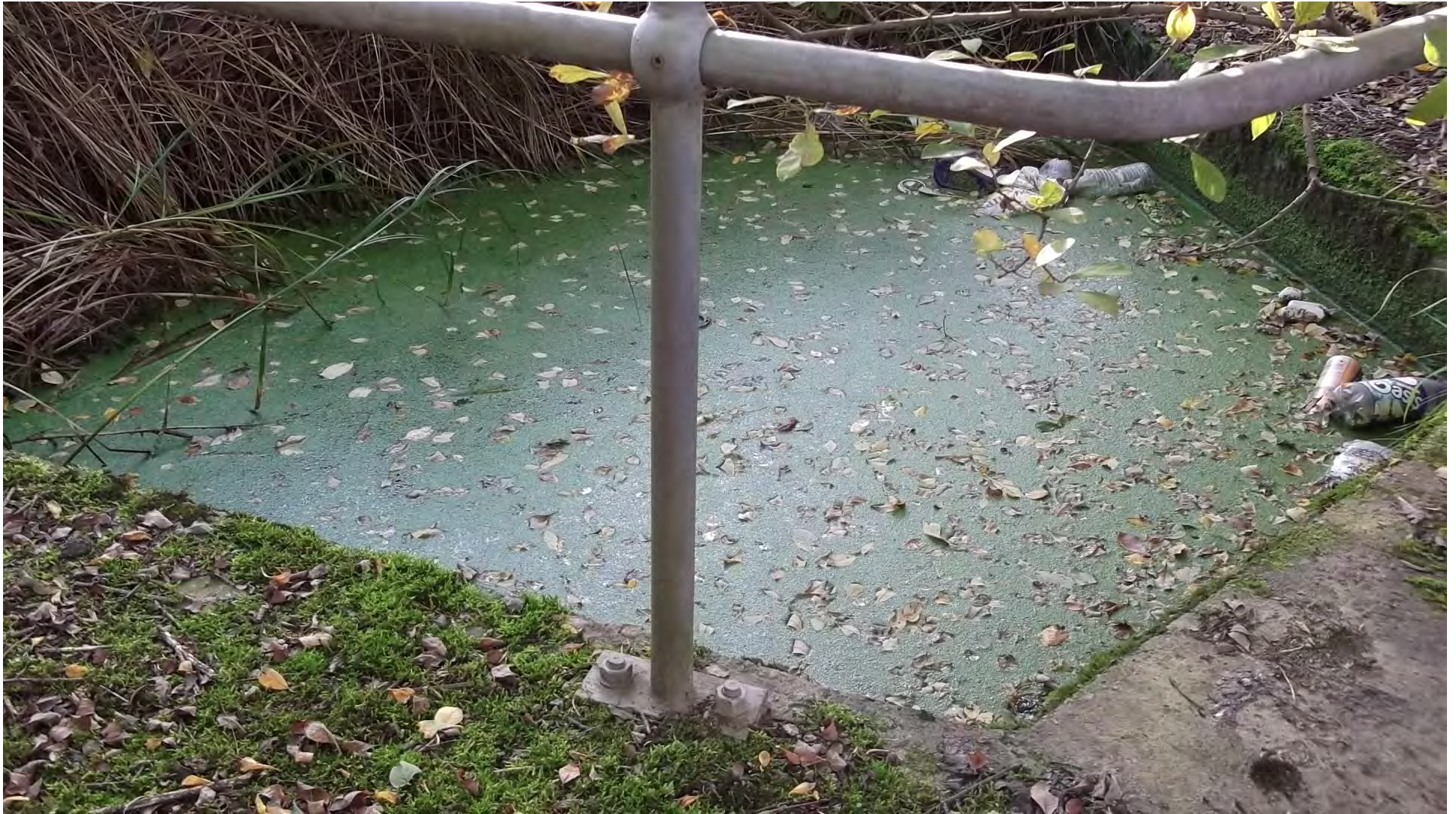
Photograph 30 –Blocked culvert inlet on the eastern side of the Weighbridge Road, north of the site.
