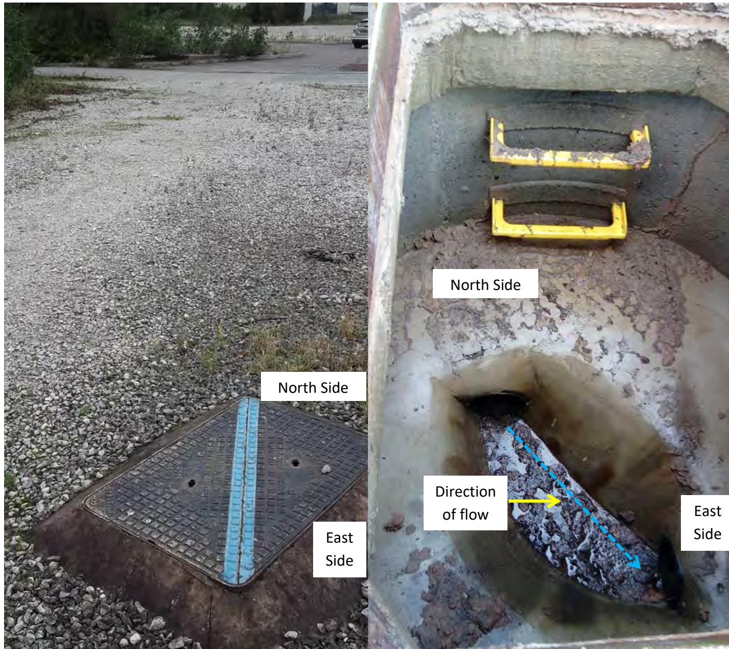
Photograph 10 –Surface water manhole located to the south side at the top of the site access ramp. Surface water inlet drains from the north and proceeds eastwards.
