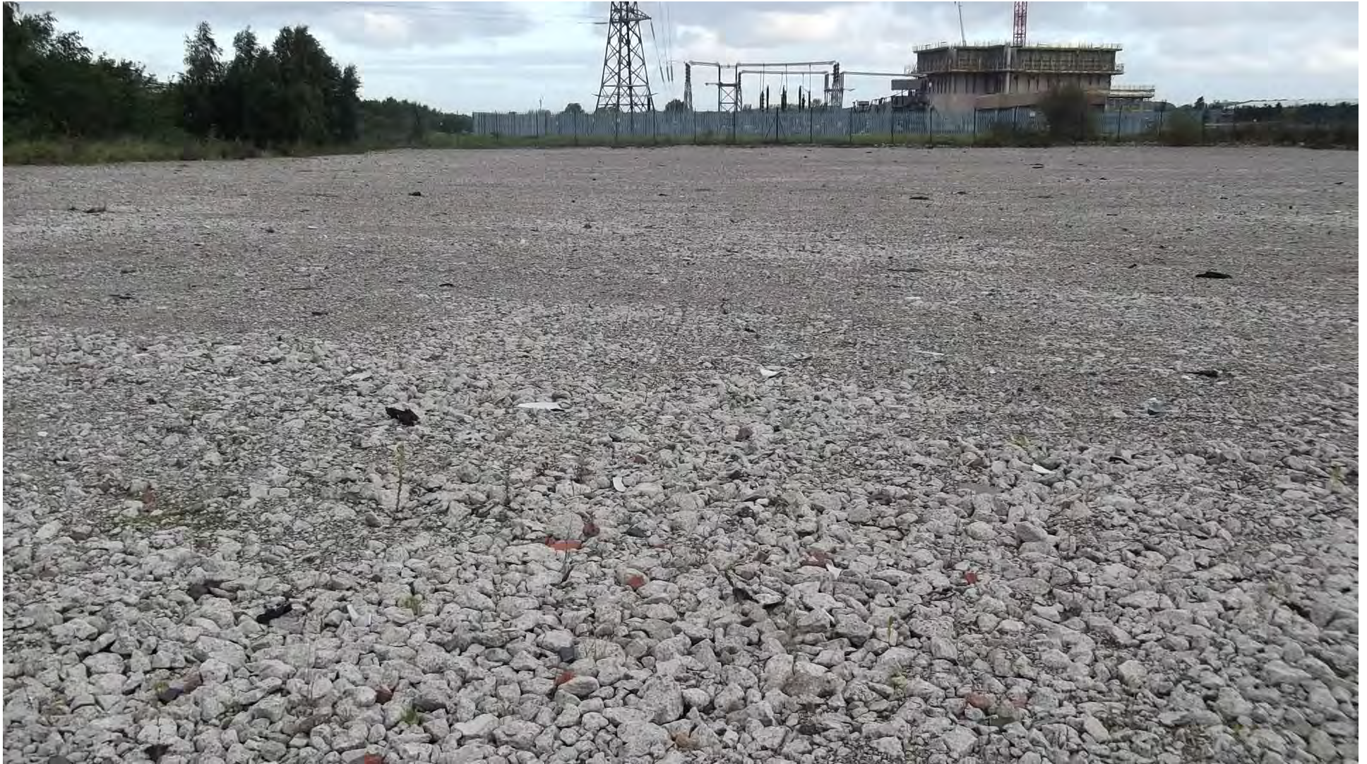
Photograph 17 – Looking northwards on to demolished hard-core area of Shotton Power Station. Construction of new EfW facility and operational sub-station in background.
