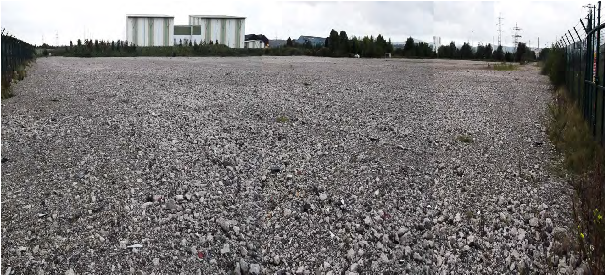
Photograph 19 – Looking south-westwards on to the demolish hard-core area of Shotton Power Station at the eastern boundary of the site. Flintshire Bridge Site 400kv Converter Station in background.
