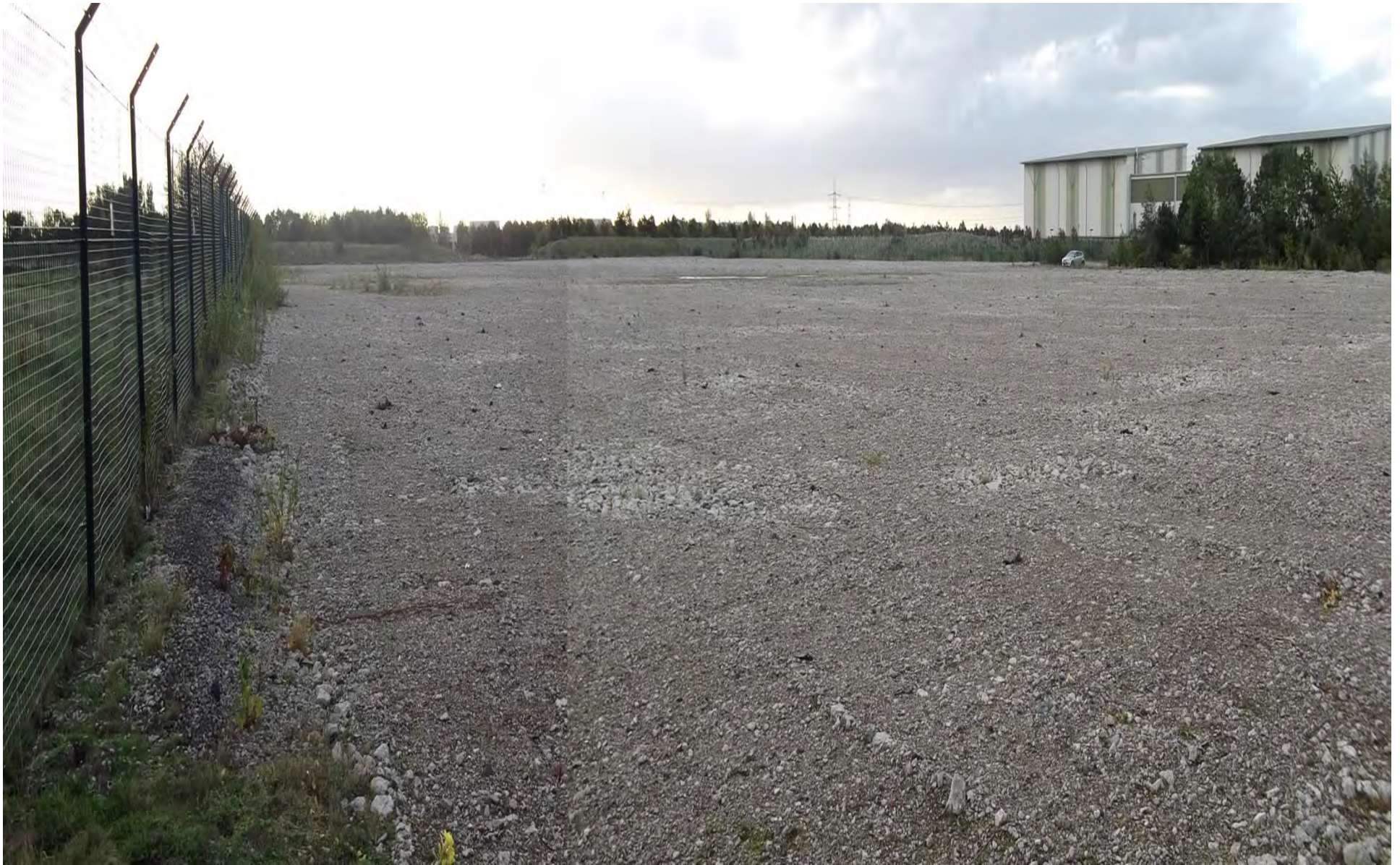
Photograph 18 – Looking south-eastwards on to demolish Shotton Power Station at north-western corner of site.
