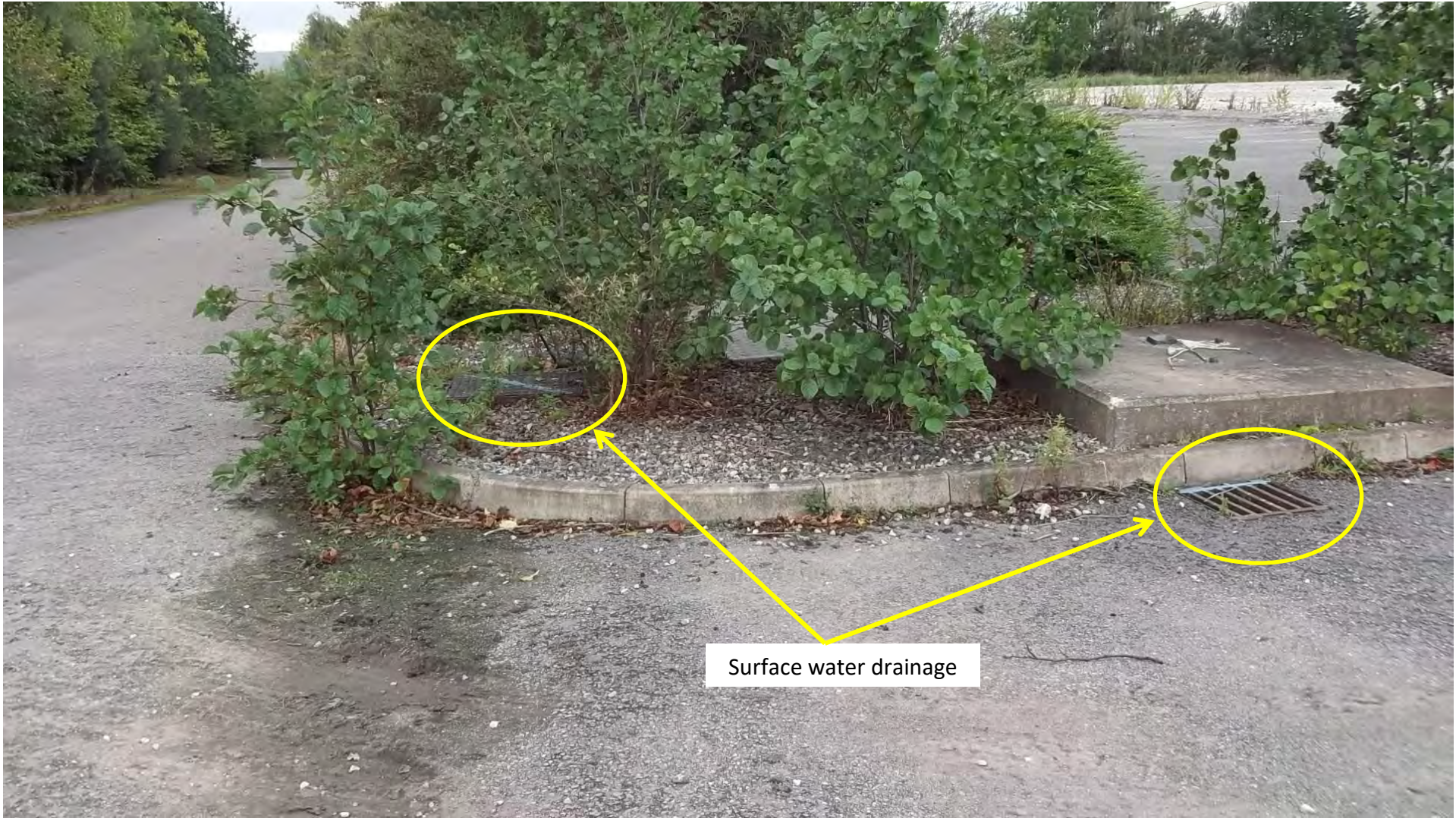
Photograph 1 – Looking westwards down site access ramp and onto car park area. Surface water drainage present along site access ramp and car park.
