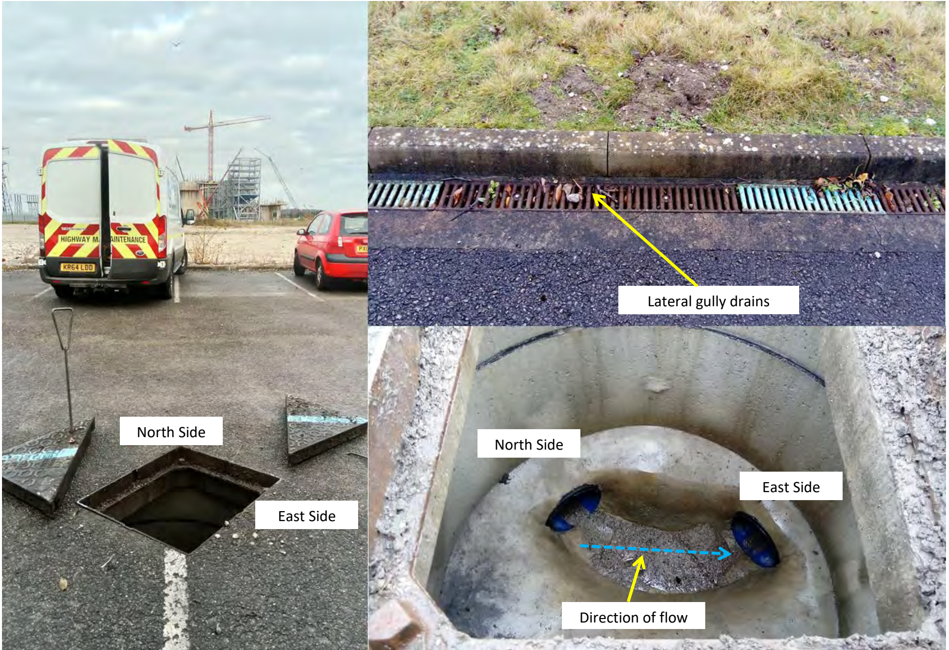
Photograph 4 – Surface water drainage in carpark. Lateral gully drains present along the southern edge of car park draining eastwards. Manhole receiving surface water from the north and proceeding eastwards.
