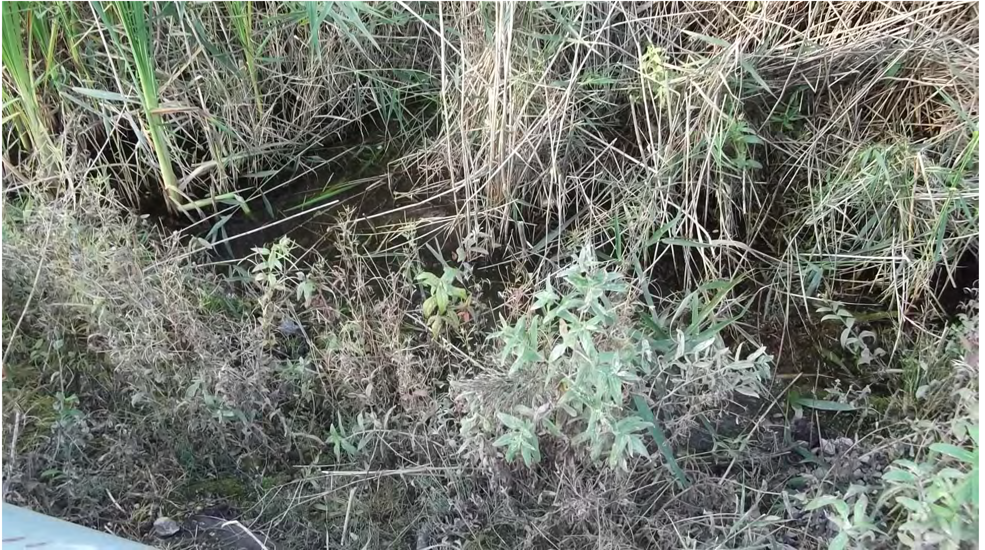
Photograph 31 –Blocked culvert outlet on the eastern side of the Weighbridge Road, north of the site.
