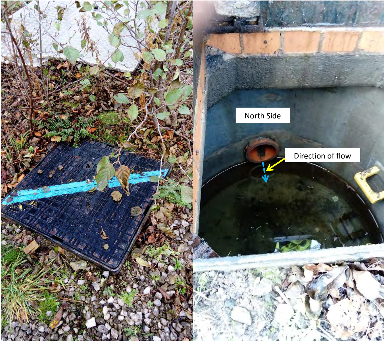
Photograph 2 – Manhole for surface water drainage at depicted in Photo 1. No outlet pipe identified, incoming pipe from the north.
