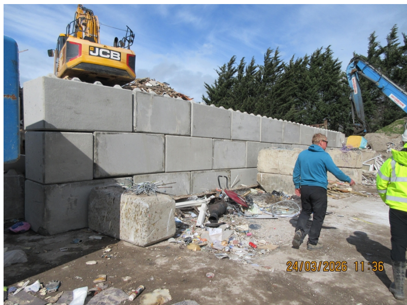
Photograph 2 - Mixed wood waste within their new concrete bay.
