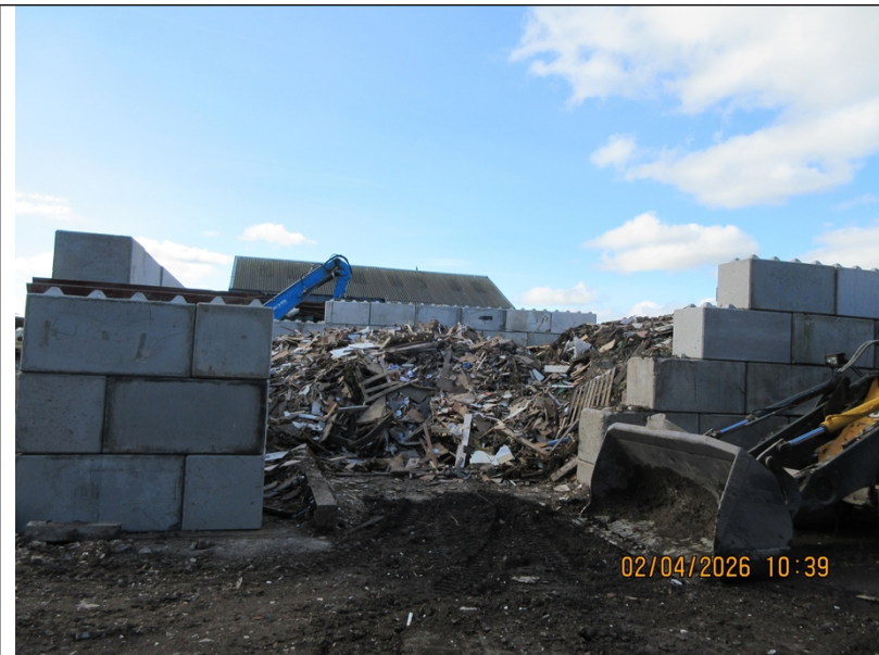
Photograph 3 - Wood waste within bay.
