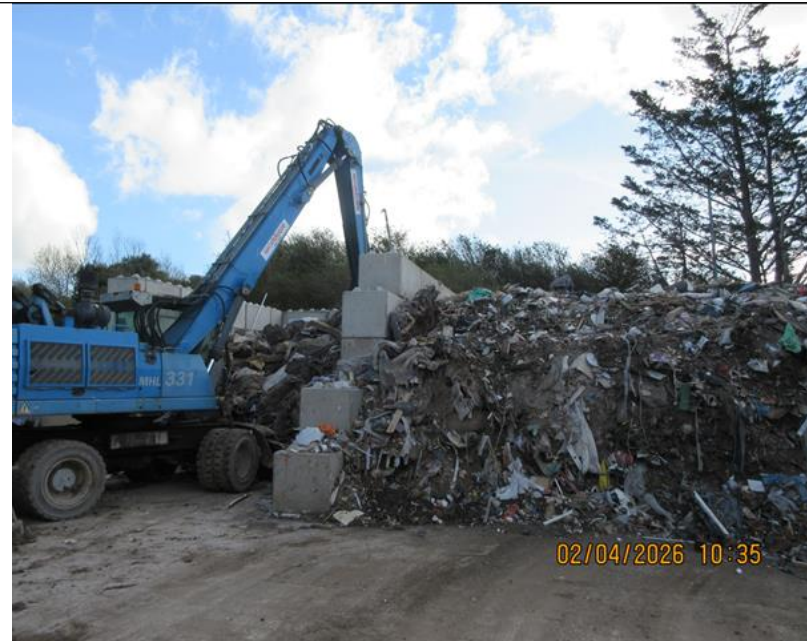
Photograph 5 - 1 metre freeboard space at the top of the mixed skip waste stockpile.
