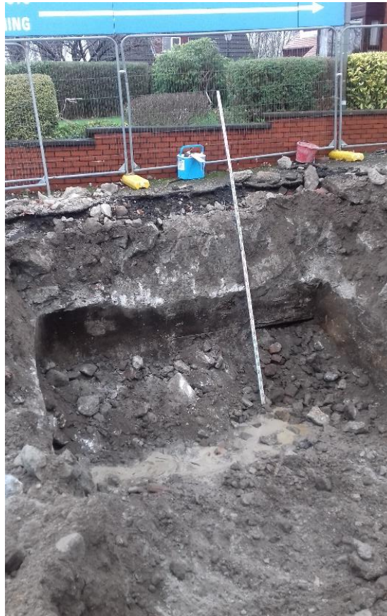
Figure 1. Image of tank validation. The concrete cradle has been retained for structural reasons.
