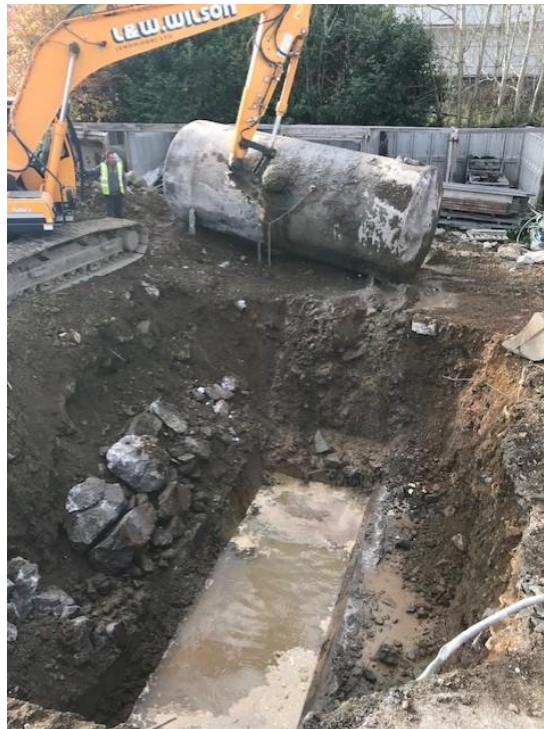
Figure H. Beware of bad practise! A dangerous tank removal in progress with tank contents leaking into the environment after removal.
