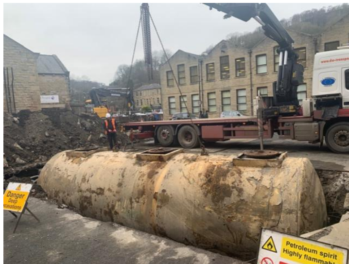
Figure G. The safe removal of a historic tank from the ground after excavation.
