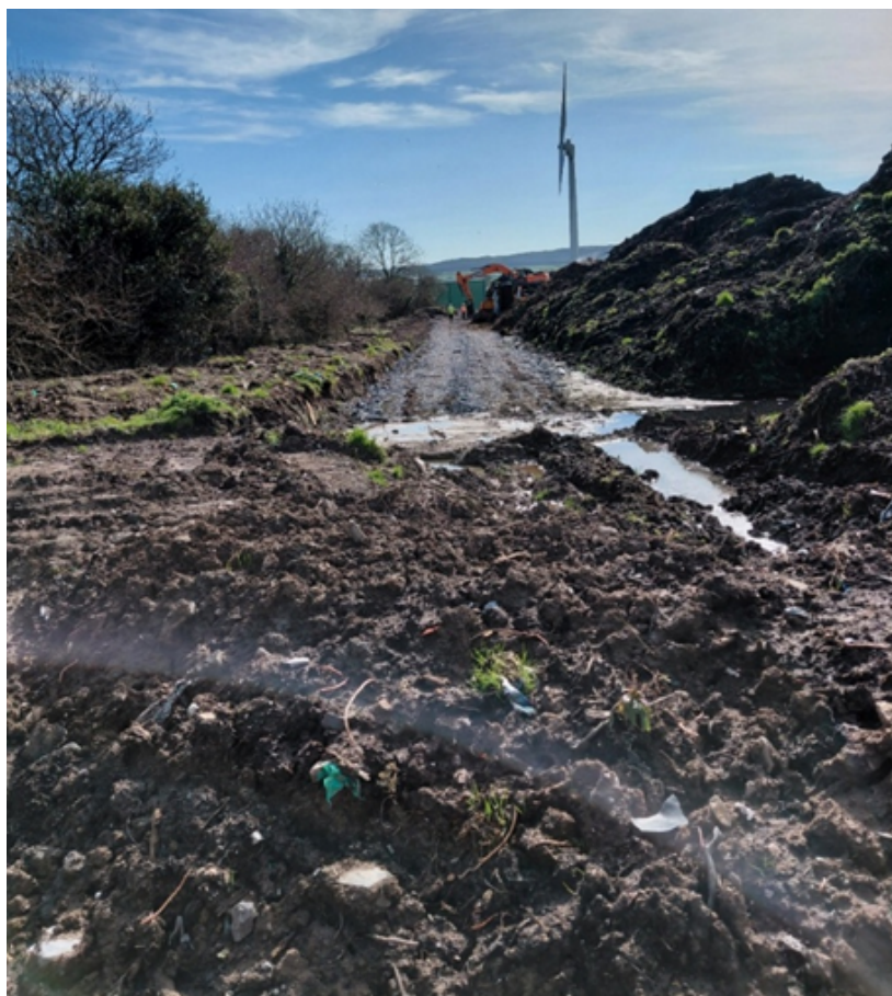
Figure 18 Photo showing newly installed hard standing access path to east of compost pad.
