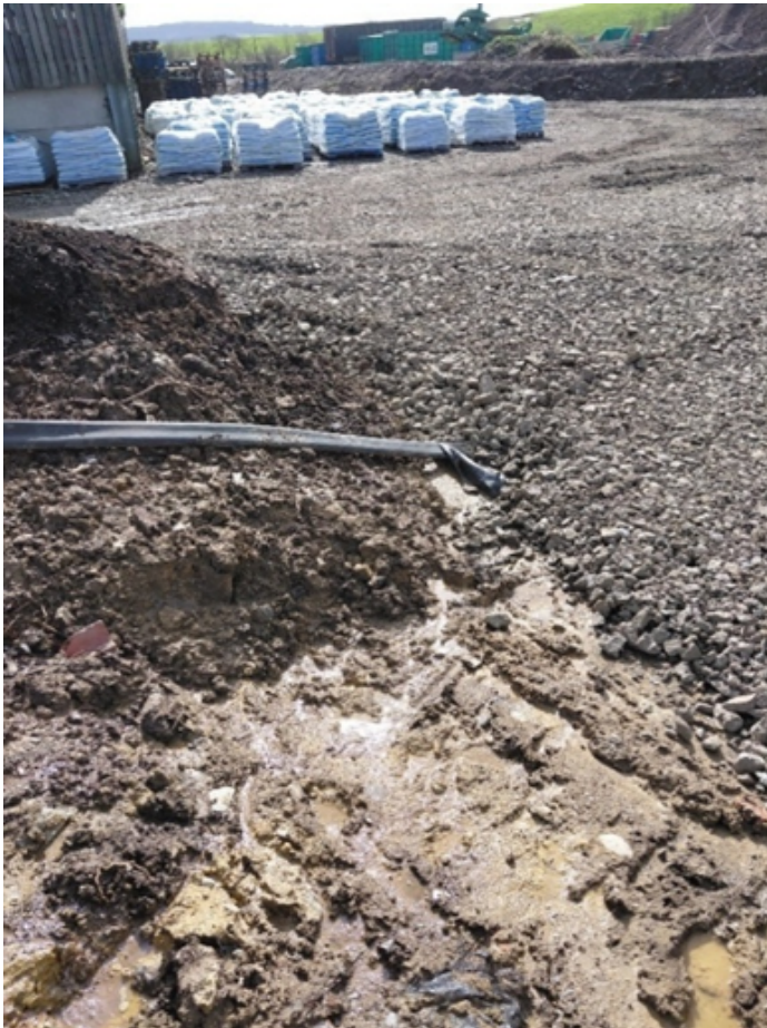
Figure 19 Photo showing crushed fire water pipe emerging from newly installed hardstanding.
