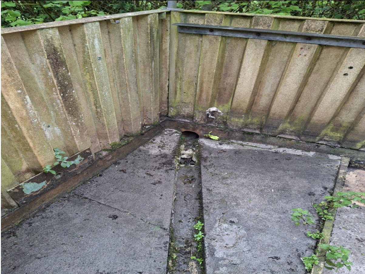
Figure 1 Crack in the concrete base of the Storm Discharge channel.
