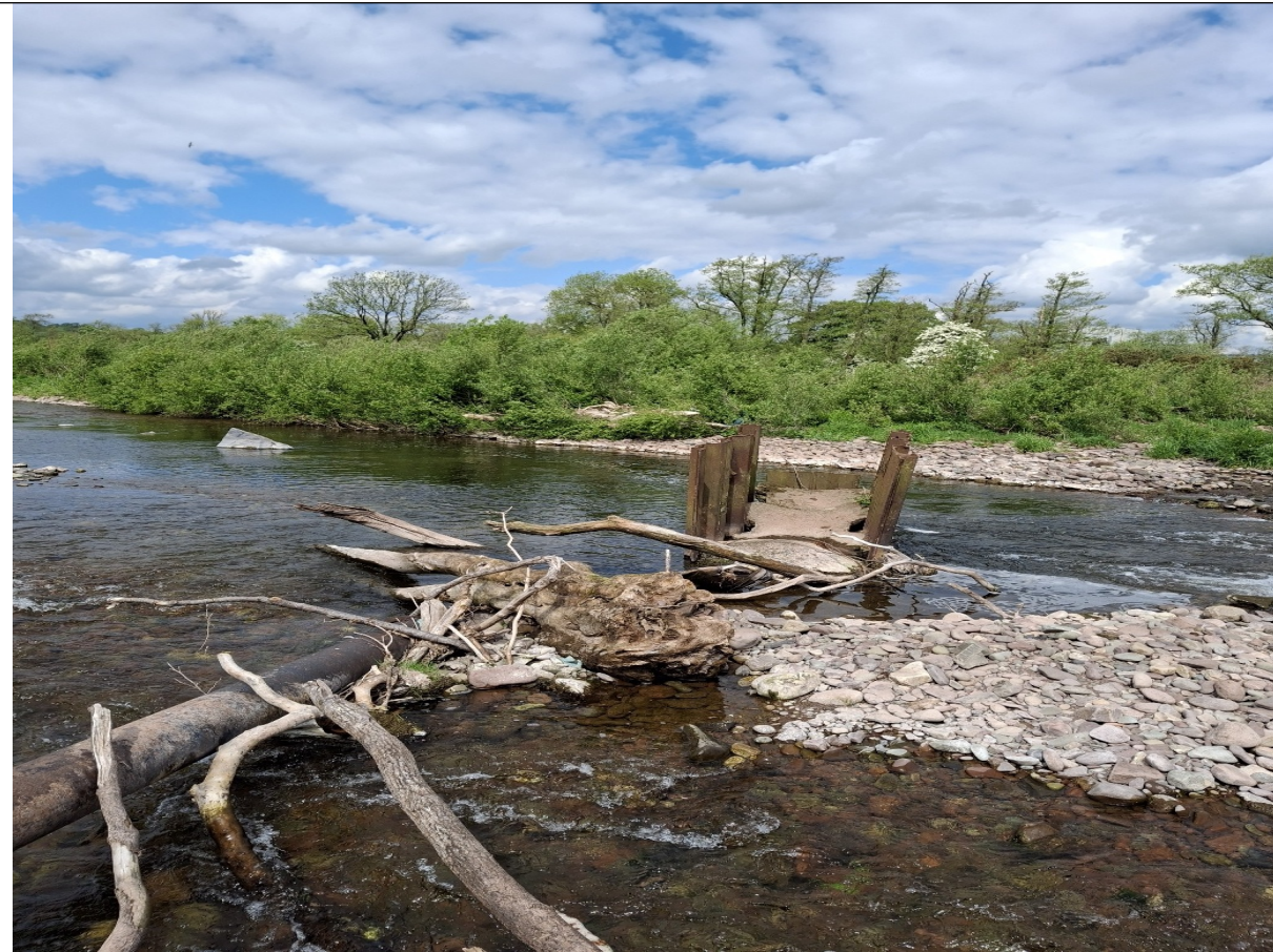
Figure 3 Broken pipe and old headwall in the middle of the Afon Sawdde
