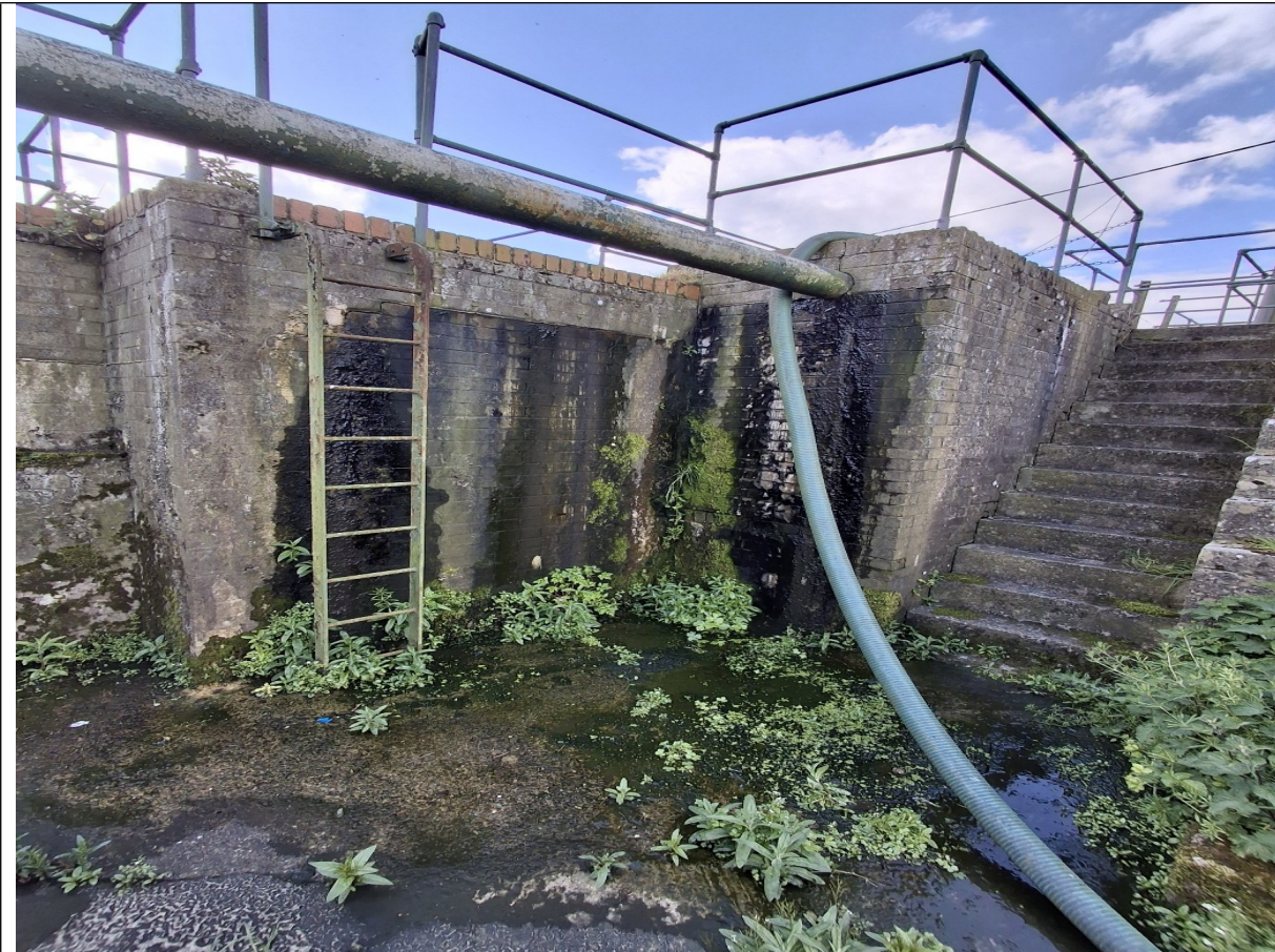
Figure 1 Leak from crack in the splitting chamber for filter beds 1 and 2, pooling on the ground
