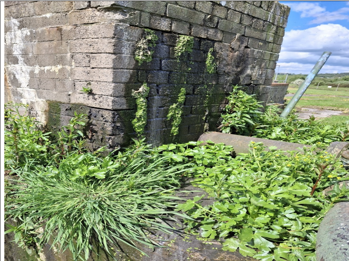
Figure 2 Leak from cracks in the distribution chamber for filter bed 3, grey fungus present on ground at the base of chamber
