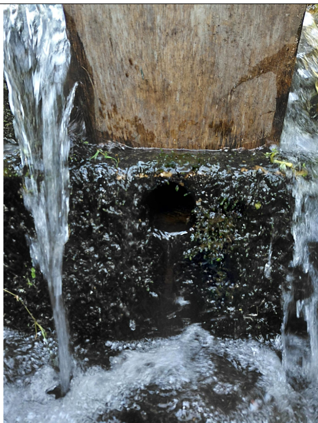
Figure 2: No water flowing through the hands-off flow outlet.
