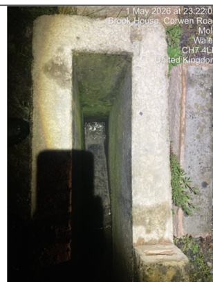
Figure 2 – Inlet flows returned to normal once blockage was cleared
