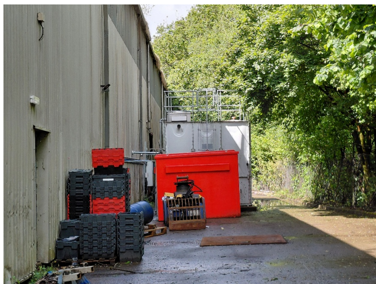
Photo 4 - Water tank for water cannon/heat detector system
