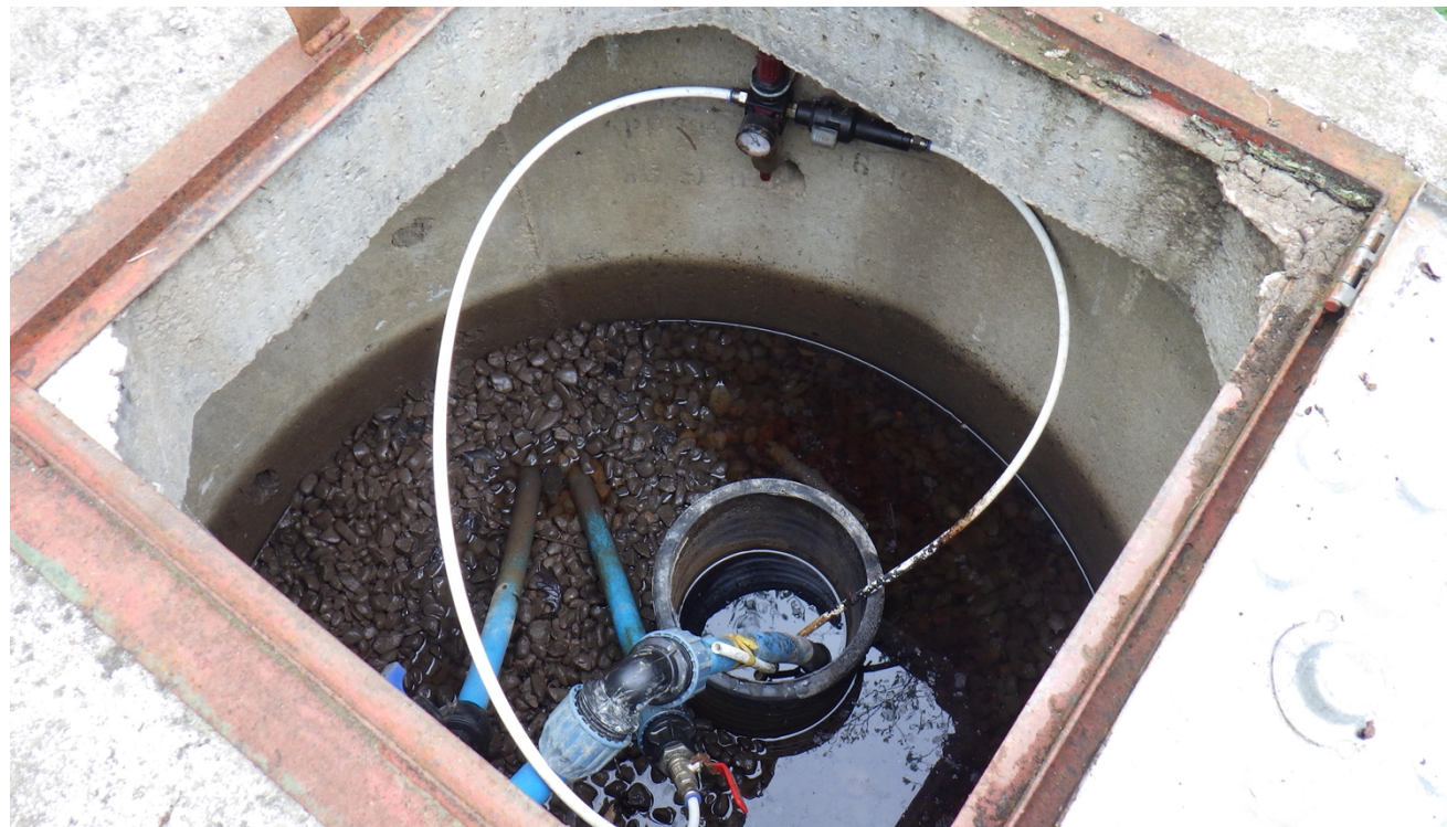
Photograph showing sump 5 following intervention by staff
