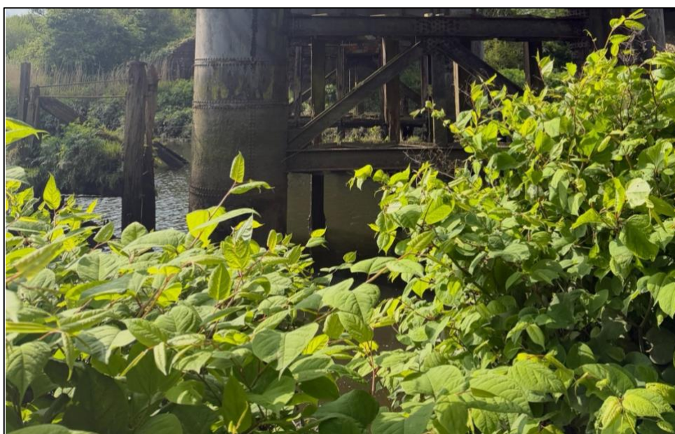
Figure 6: Japanese knotweed beneath structure
