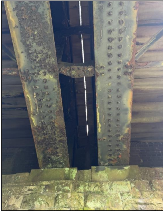
Figure 7: Sections of steelwork requiring replacement
