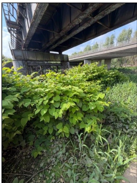
Figure 4: Japanese knotweed beneath structure
