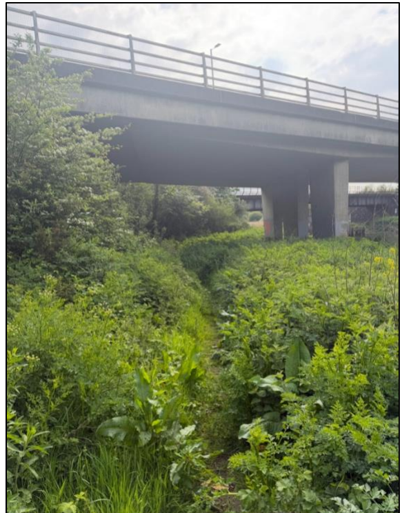
Figure 10: Overview of survey area
