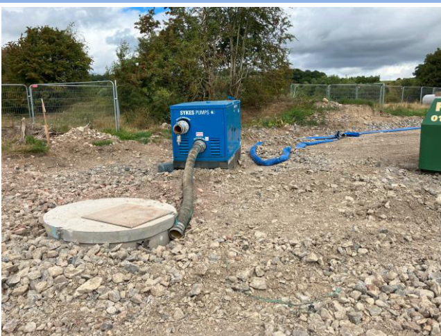
Photograph 5: Drainage pump in road area
