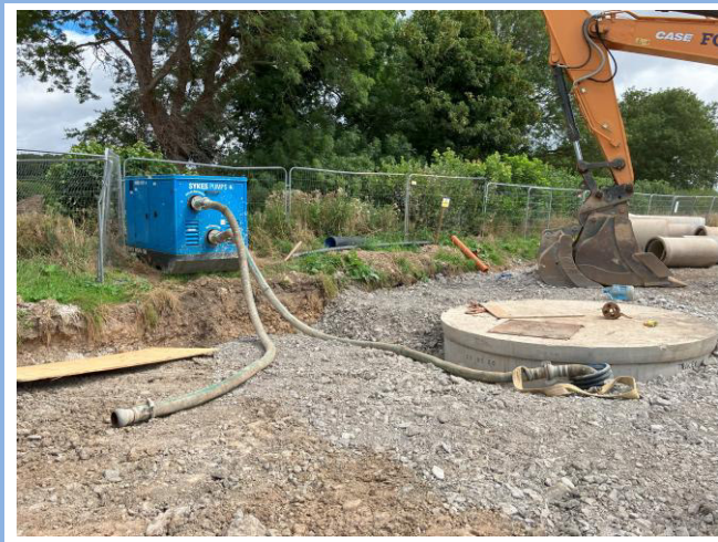
Photograph 13: Drainage pump in northern site boundary
