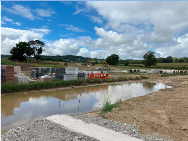
Photograph 5: Waterlogging in central site area
