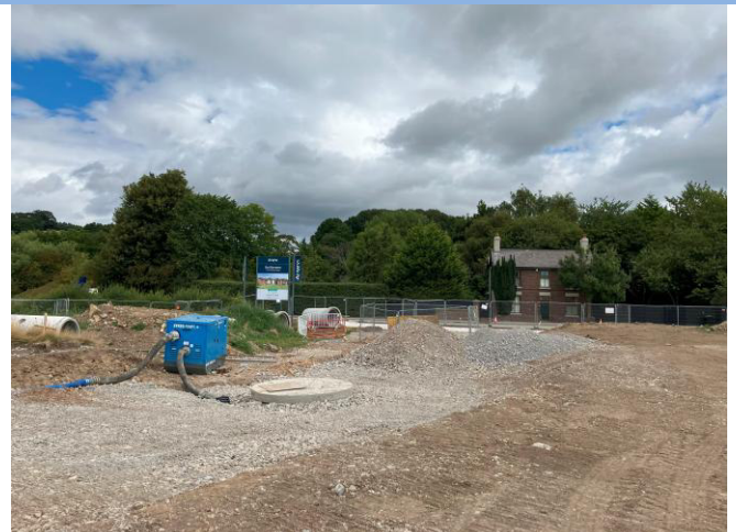
Photograph 6: Drainage pump in road area
