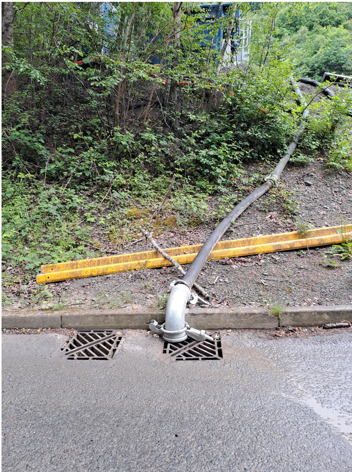
Figure 3 – The silt buster outlet pipe discharging to a road drain as observed during the visit.
