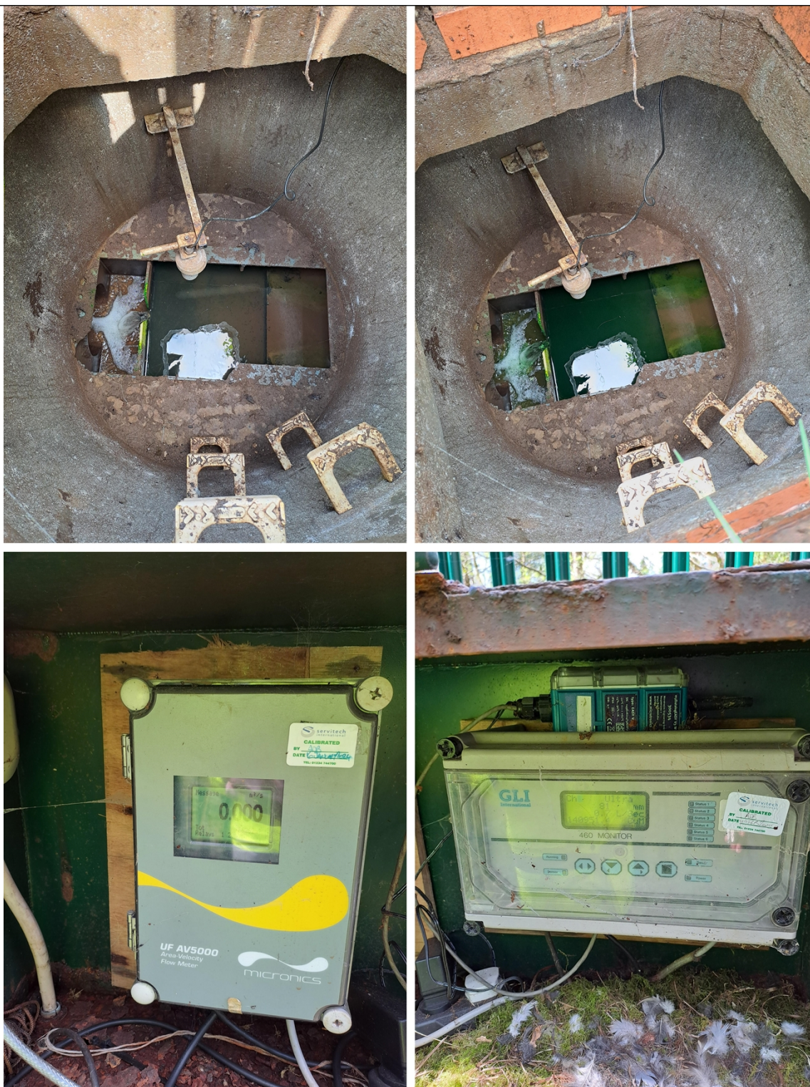
Figure 4 – Evidence to support that site drainage is discharging to the DCWW foul network and not via the permitted point.
