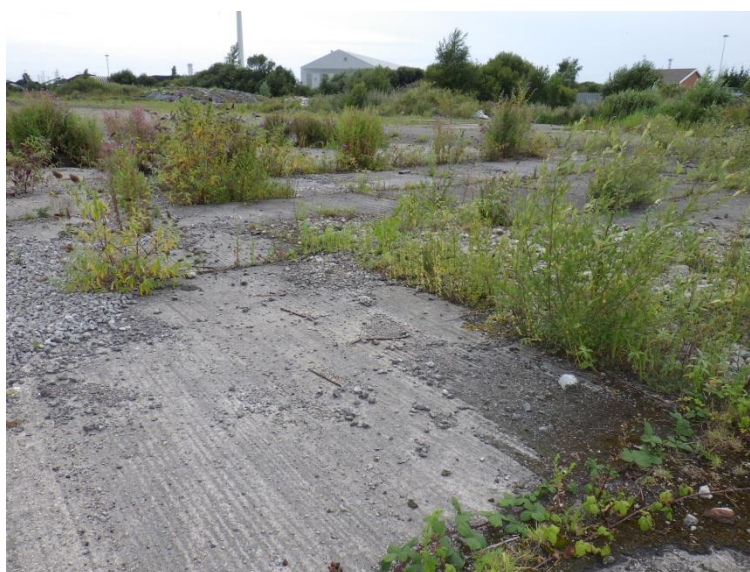
Photograph 5. Poorly drained hard-standing in north of study area, with ruderal community establishing in cracks
