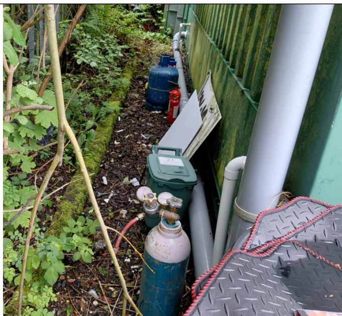
Photograph 2. Gas canisters on site hidden behind the staff cabin
