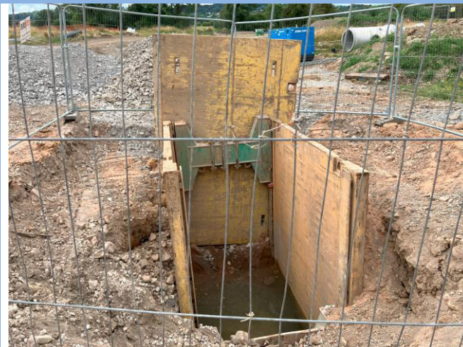
Photograph 9: Low water levels in drainage area
