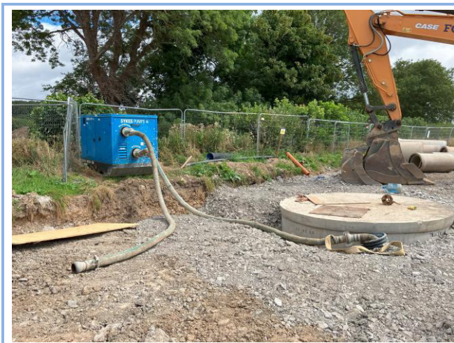
Photograph 13: Drainage pump in northern site boundary
