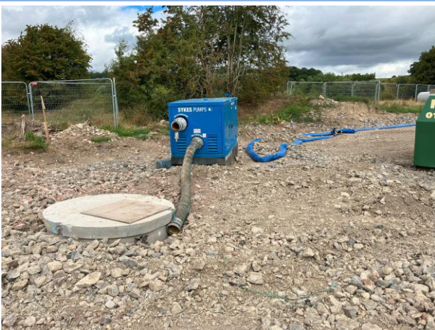
Photograph 5: Drainage pump in road area
