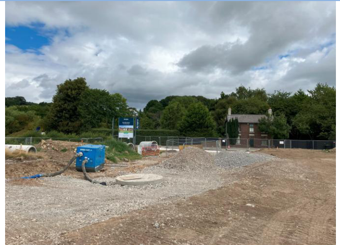
Photograph 6: Drainage pump in road area
