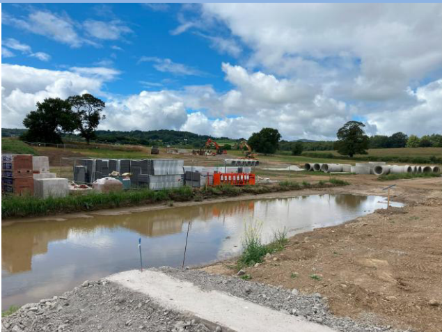
Photograph 5: Waterlogging in central site area
