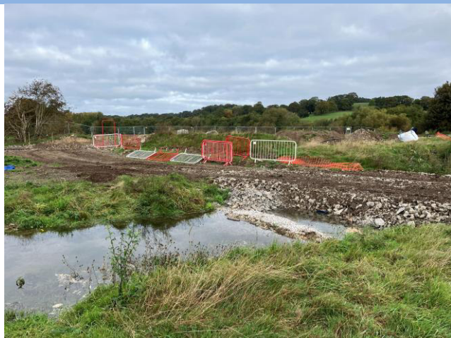
Photograph 11: Water filtration area
