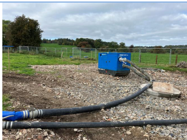
Photograph 13: Pump 2 in southern road area
