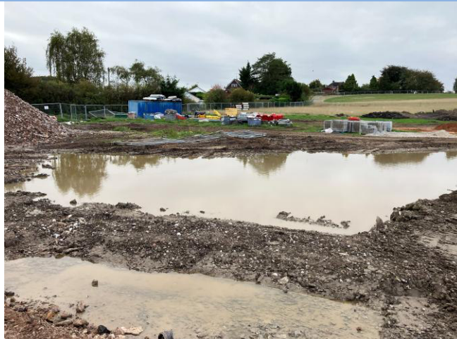
Photograph 14: Waterlogging in northeastern site area
