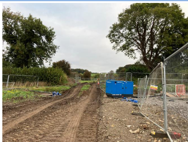
Photograph 7: Pump in northern area next to link road
