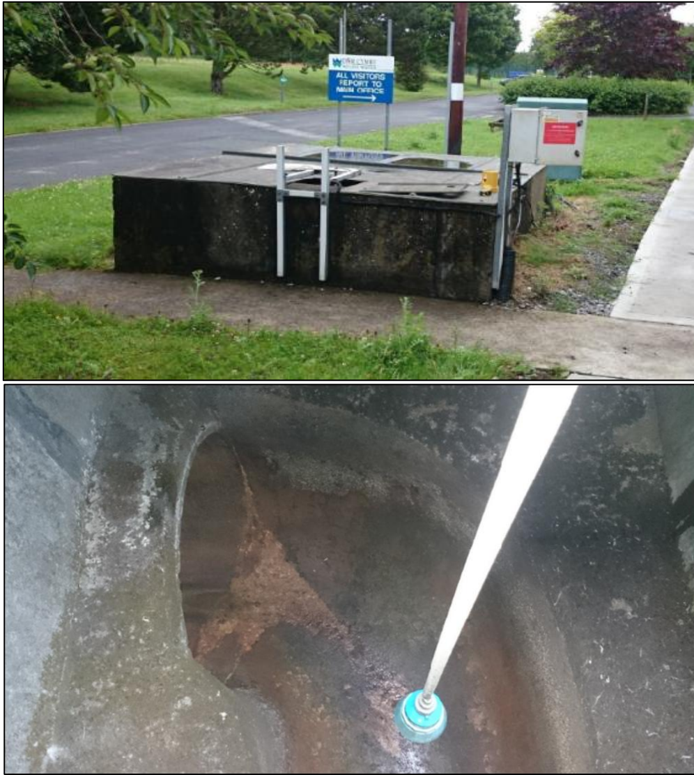
Figure 6: EDME Monitoring Chamber for Settled and Screened Discharge.
