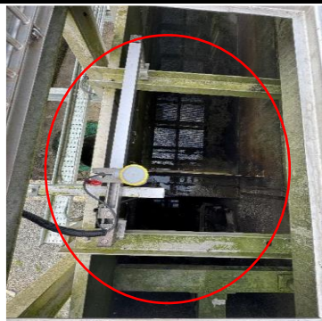
Figure 5: EDMS Monitoring to Storm Storage Tank Split.
