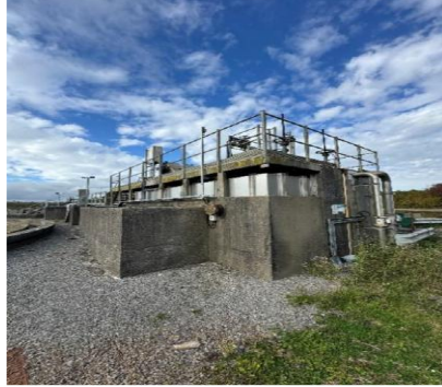
Figure 4: Gowerton Headworks Splitter chamber.
