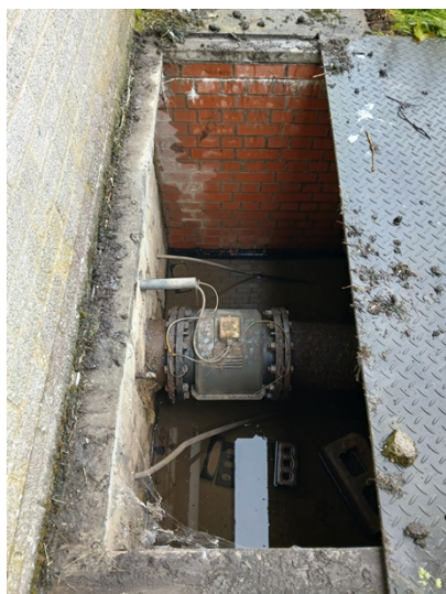
Fig 3 - Flow meter with telemetry located to the rear of Dwr Cymru pumping station
