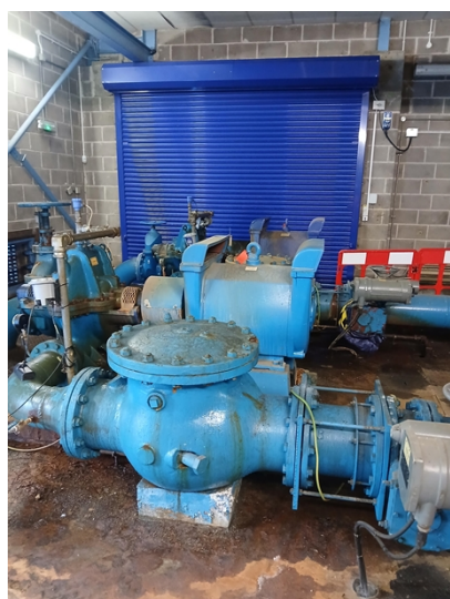
Fig 5 - Interior of Dwr Cymru pumping station
