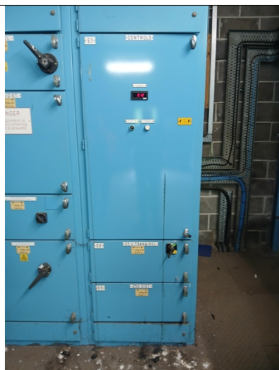
Fig 4 - Interior of Dwr Cymru pumping station
