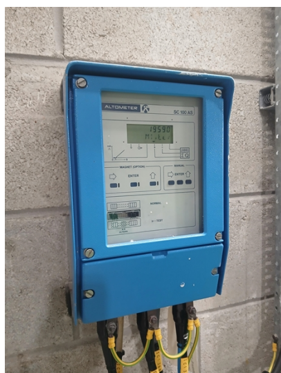
Fig 3 - Meter readouts clearly visible
