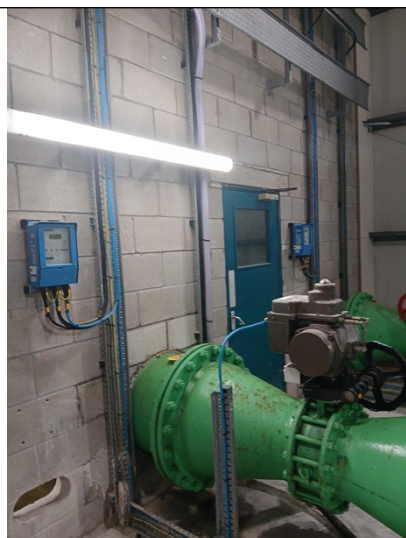
Fig 2 - Flow meter heads/Control panel displays
